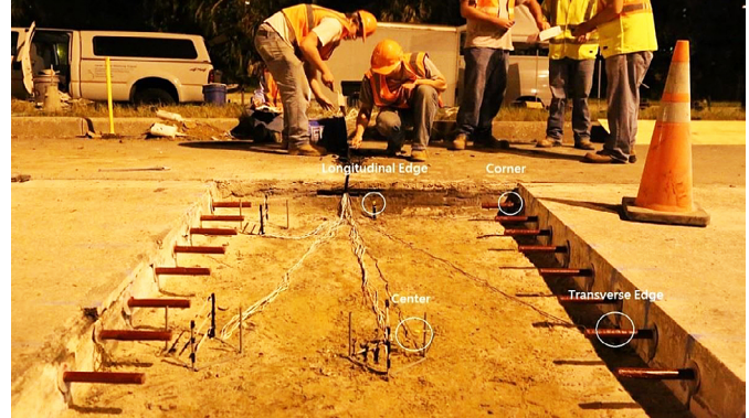
Researchers set temperature sensors in four locations in the space prepared to receive a replacement slab.
