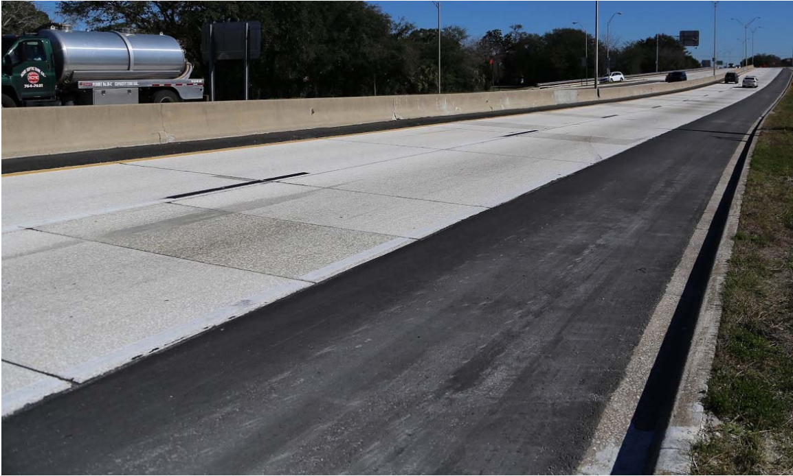
Figure 6-12. Picture of the replaced slab and neighboring slabs in the first field study taken on 1/20/14.
