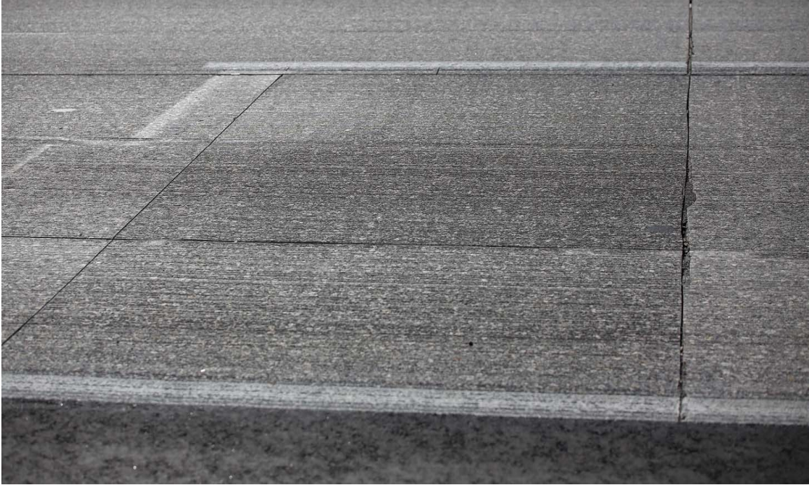
Figure 6-18. Picture of the replaced concrete slab in the second field study taken on 1/20/14.
