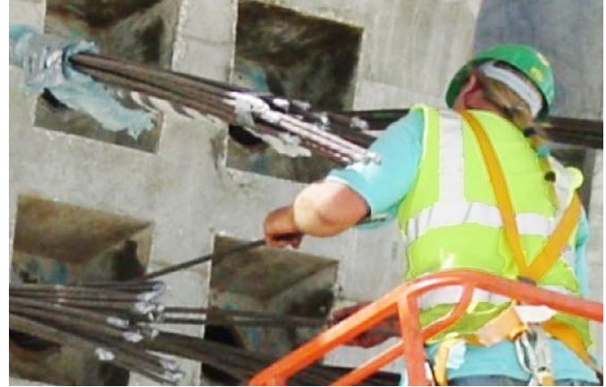
A worker places post tensioning strands in the ducts cast into this bridge component.
