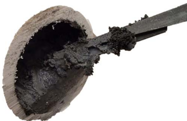
Figure 109—PT4-6 soft grout
