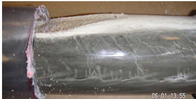
Figure 63—White grout at 12:00 position and darker grout everywhere else in tube injected with material C675
