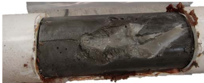
Figure 117—Soft grout located in segregation canal
