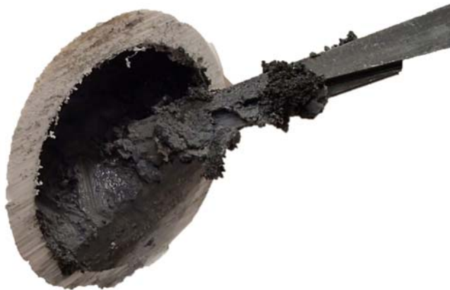
Figure 109—PT4-6 soft grout
