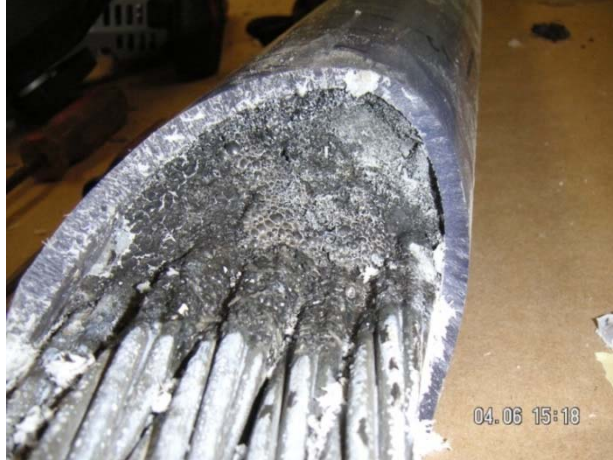
Figure 56—Grout containing air bubbles found at top of tubes containing PT4-1 mixed at MWD
