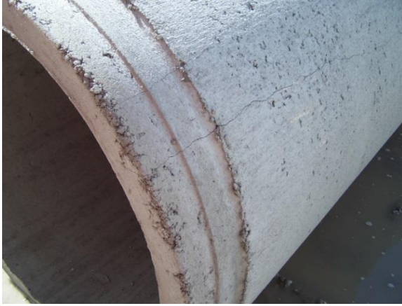
Figure 3-11: Hairline Crack on RCP
