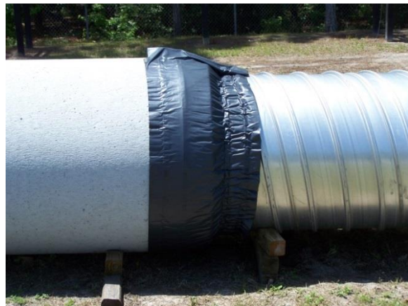
Figure 3-16: Dissimilar Pipe Coupler at RCP-to-CMP Junction
