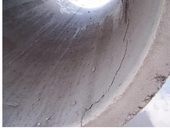
Figure 3-12: Larger Crack on RCP
