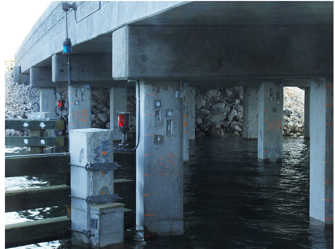
Bridge and fender piles of the Key Royale bridge are marked with access points of embedded instruments.
