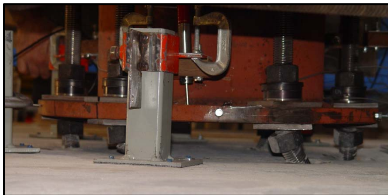
Figure 5-8. FS1 anchor bolts in failed condition
