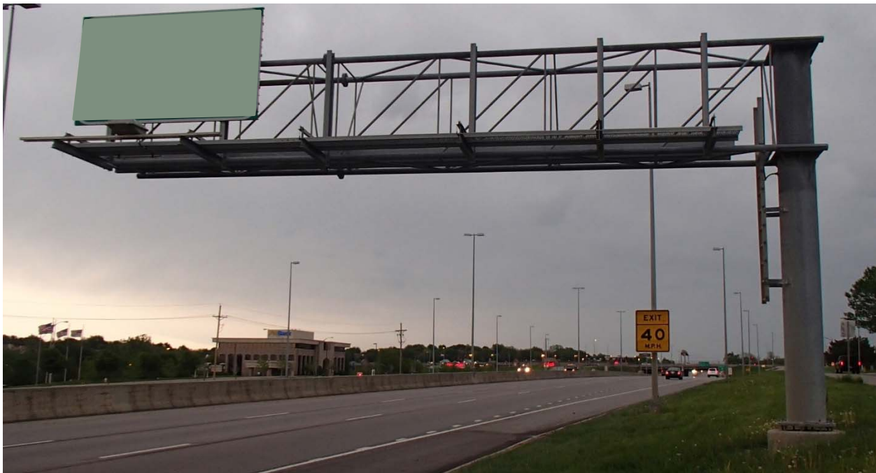
Figure 1-1. Cantilever sign structure with an ungrouted stand-off base plate
