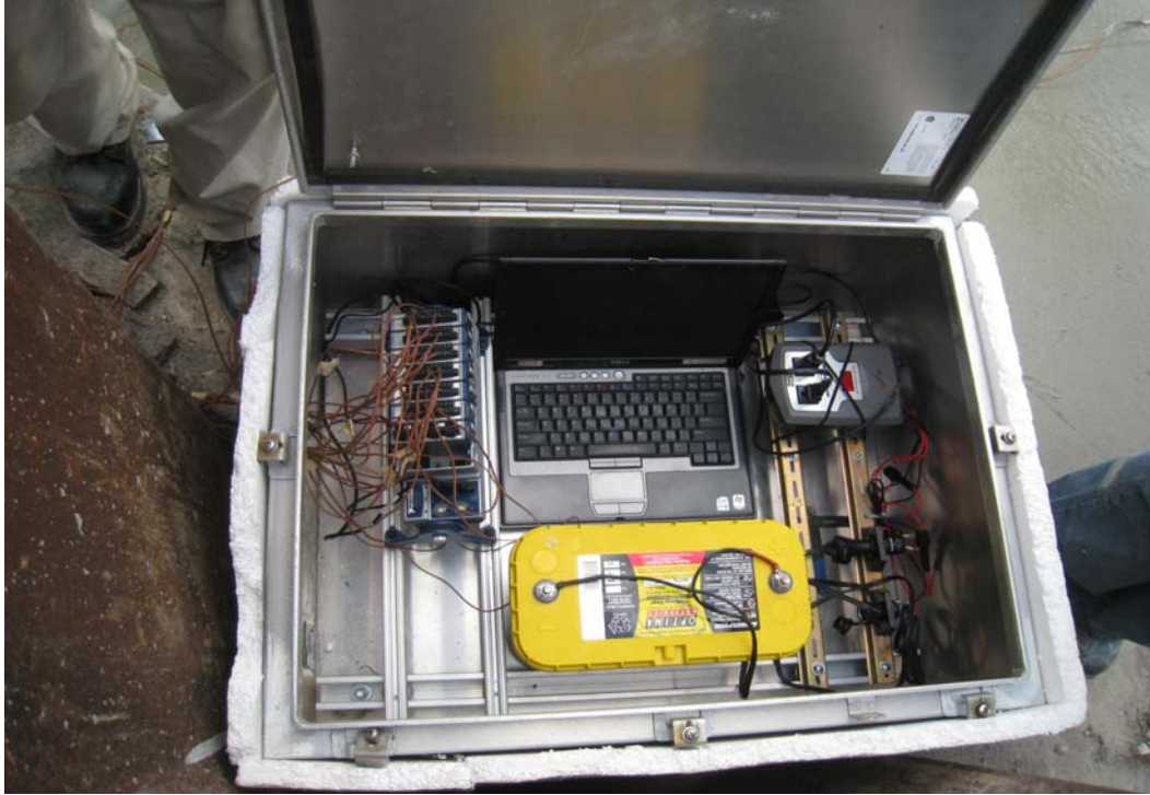
Figure 5-5. Data acquisition equipment with thermocouple wiring.
