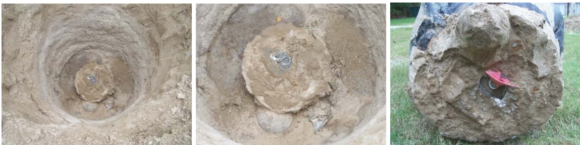
Figure 4-8: Poor contact between the tip grout bulb (left two photos) and bottom of shaft (right photo)
