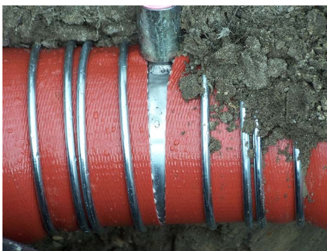
Figure 3-4: No leaks observed during initial test of improved membrane seal design
