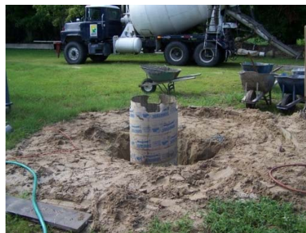
Figure 2-16: Failed Sonotube during removal
