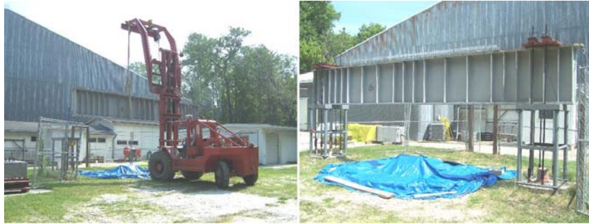
Figure 2-66: Setup reaction system for static load test
