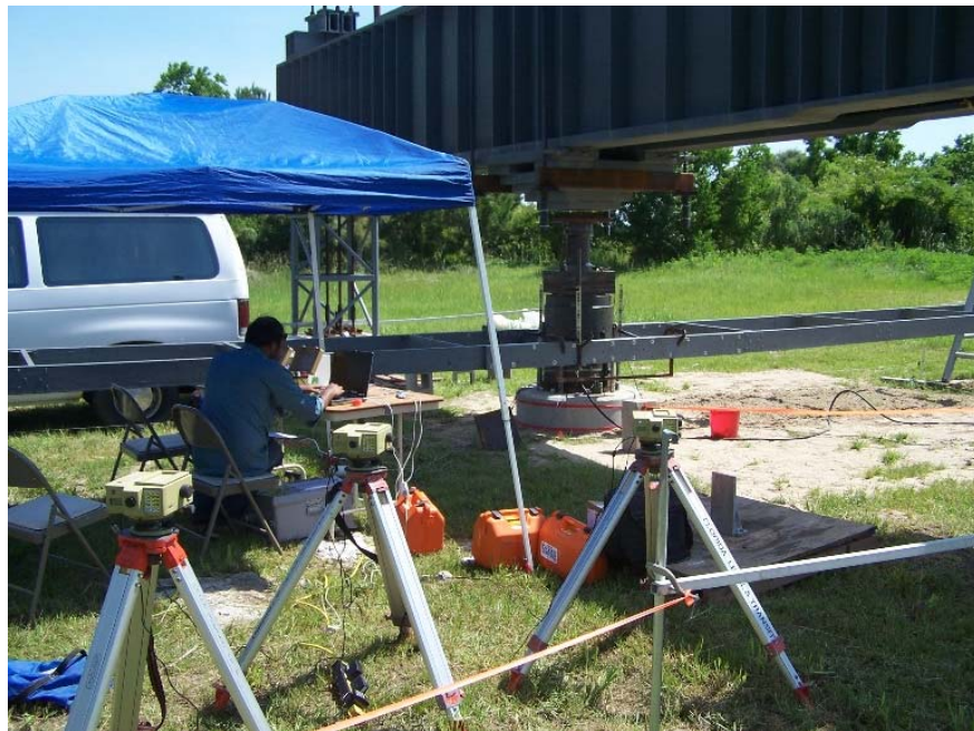
Figure 3-68: Digital levels used to monitor shaft and wooden frame displacements
