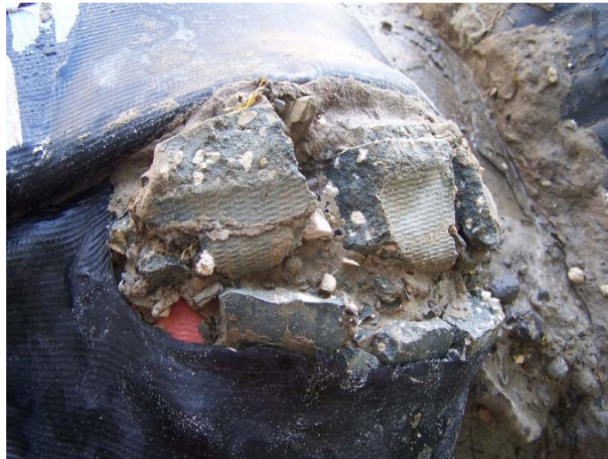
Figure 4-10: Side membrane pierced by concrete between seal and side membrane as the bottom membrane seal expanded outwards during seal grouting
