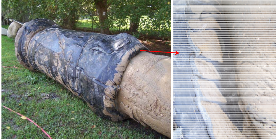
Figure 4-18: Top of side membrane failure as grout flowed upwards during side grouting of long shaft
