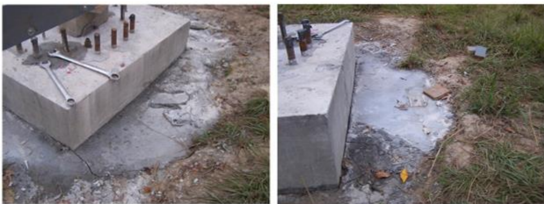
Figure 5-31. Ground surface crack (pile 2: top bag)
