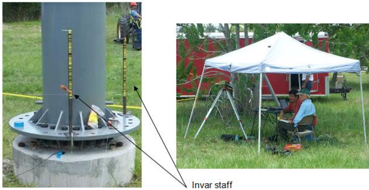
Figure 7-6. Digital level and invar staffs for vertical deformation monitoring
