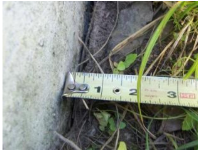
Figure 7-19. Torsional crack and gap after loading
