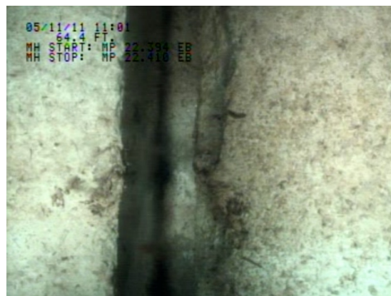
Figure 4-35. Screenshot from pipe inspection video of Site #010, showing a joint which was not repaired.
