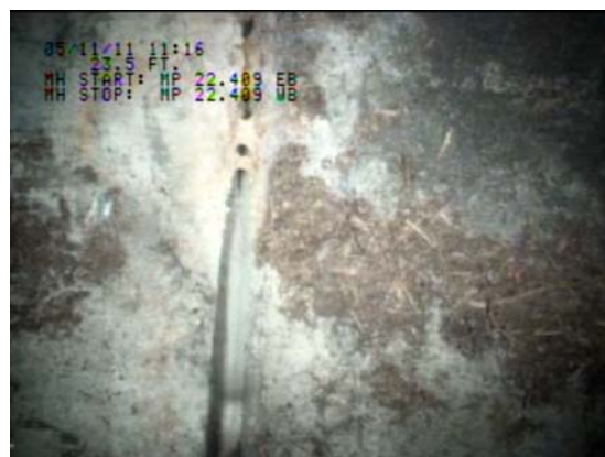
Figure 4-38. Screenshot from pipe inspection video of Site #011, showing a joint which was supposed to be repaired using an internal joint seal.
