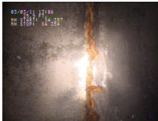
Figure 4-11. Screenshot from pipe inspection video of Site #000, showing a joint which has been repaired with chemical grout. Some remnants of the grout can be seen.
