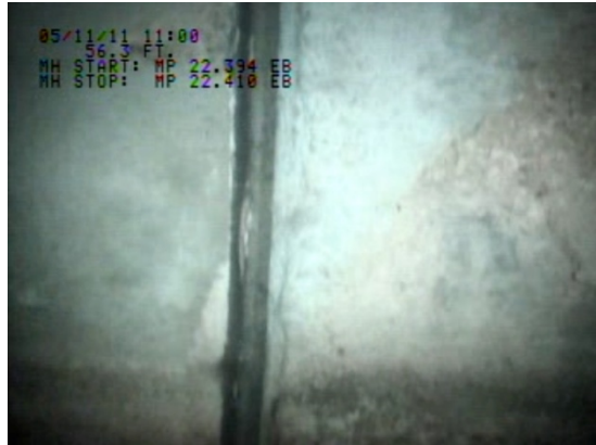
Figure 4-36. Screenshot from pipe inspection video of Site #010, showing a joint which was supposed to be repaired using an internal joint seal.
