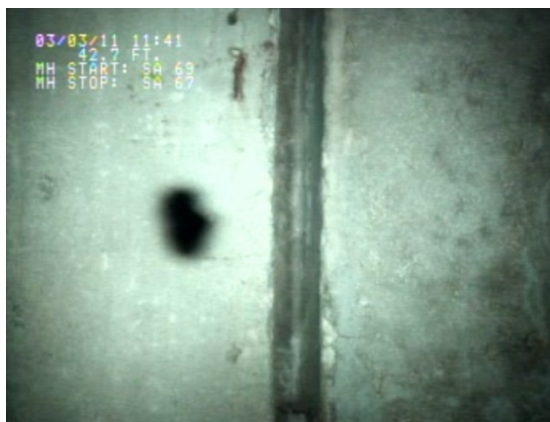
Figure 4-8. Screenshot from pipe inspection video of Site #001, showing a close up of a joint which did not show any separation and was not repaired with grout.
