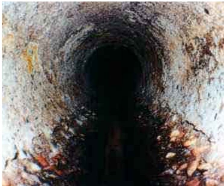
Figure 2-3. Damage from abrasive flow (Oberdorfer AG).
