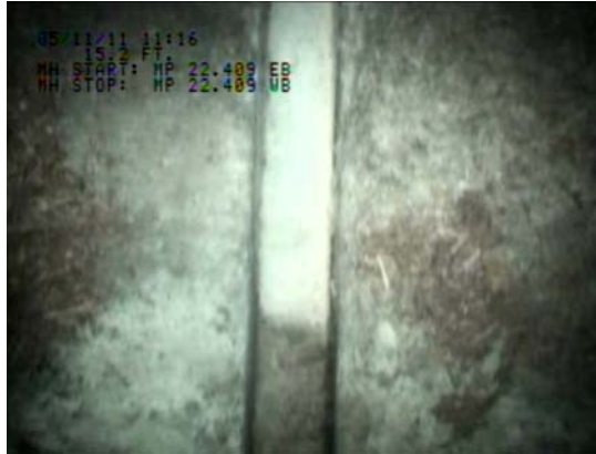
Figure 4-39. Screenshot from pipe inspection video of Site #011, showing a joint which was supposed to be repaired using an internal joint seal.
