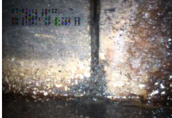
Figure 4-2. Screenshot from pipe inspection video of Site #000, showing a joint which was supposed to have been repaired with chemical grout but shows no evidence of grout.
