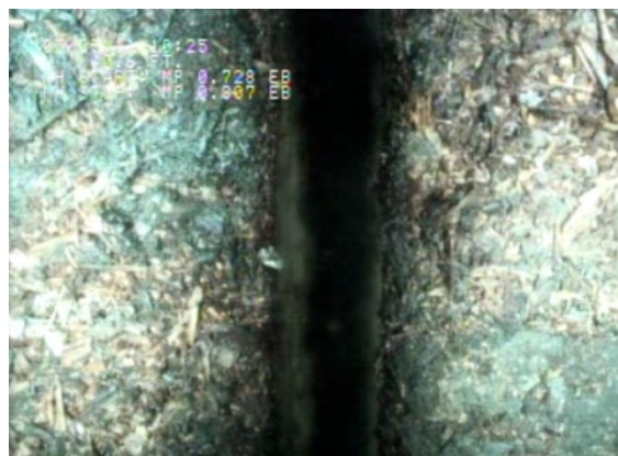
Figure 4-4. Screenshot from pipe inspection video of Site #000, showing a joint which was supposed to have been repaired with chemical grout. The orange spots may be remnants of grout.
