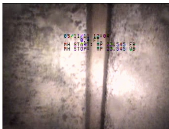
Figure 4-41. Screenshot from pipe inspection video of Site #012, showing a joint which was supposed to be repaired using an internal joint seal
