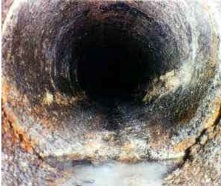
Figure 2-2. Corrosion of concrete pipe at a joint (Oberdorfer AG 2010).
