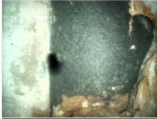
Figure 4-6. Screenshot from pipe inspection video of Site #001, showing a close up of a joint which has been repaired with chemical grout. Some remnants of the grout can be seen.
