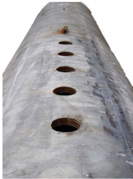
Figure 6-5. Longitudinal seam weld placed to the right of through-bolt holes. Photo courtesy of S. Dalton.
