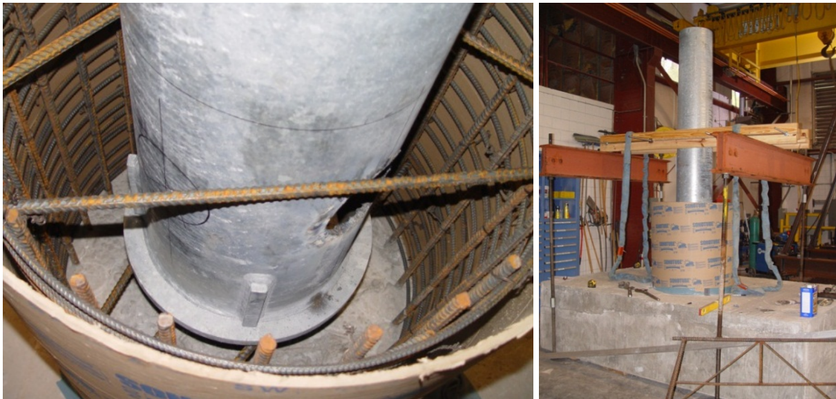
Figure 6-1. Alignment rebar within pedestal and external bracing of embedded pole. Photos courtesy of FDOT.
