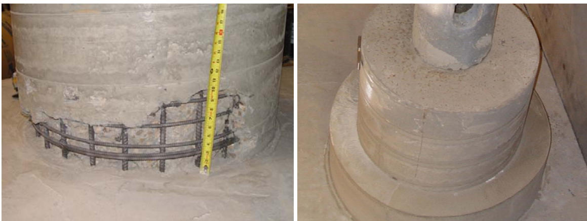
Figure 4-1. Honeycomb around pedestal and repair of pedestal. Photo courtesy of FDOT.
