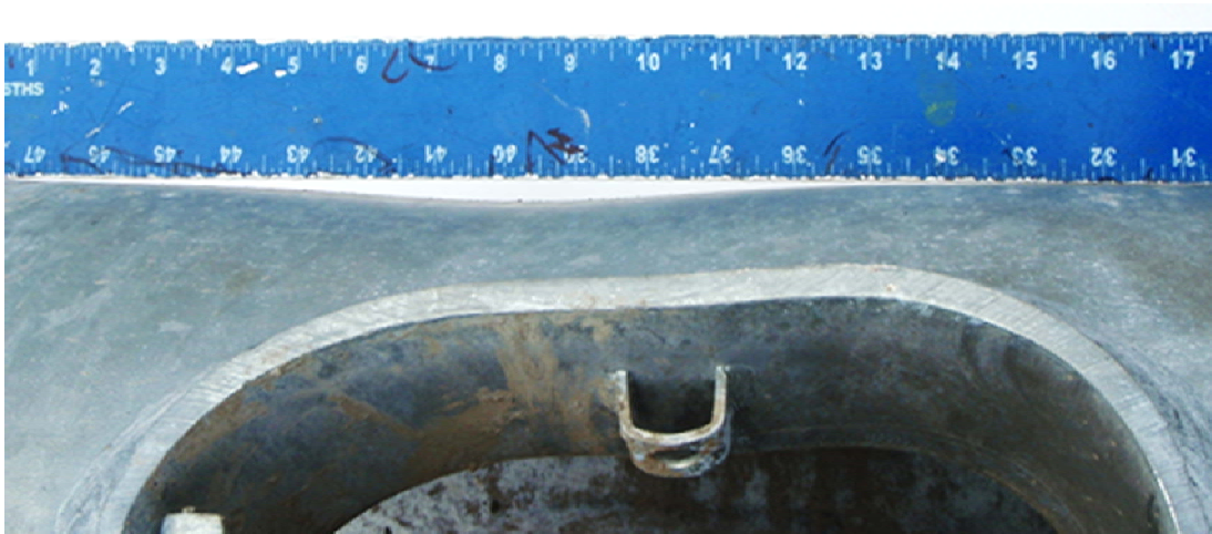
Figure 5-1. Pipe buckling near the access panel on the embedded pole. Photo courtesy of S. Dalton.
