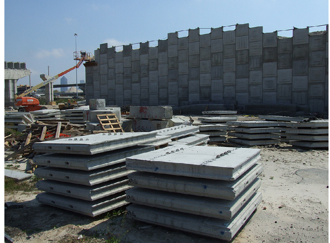
MSE wall being constructed from concrete panels for an overpass in Jacksonville.
