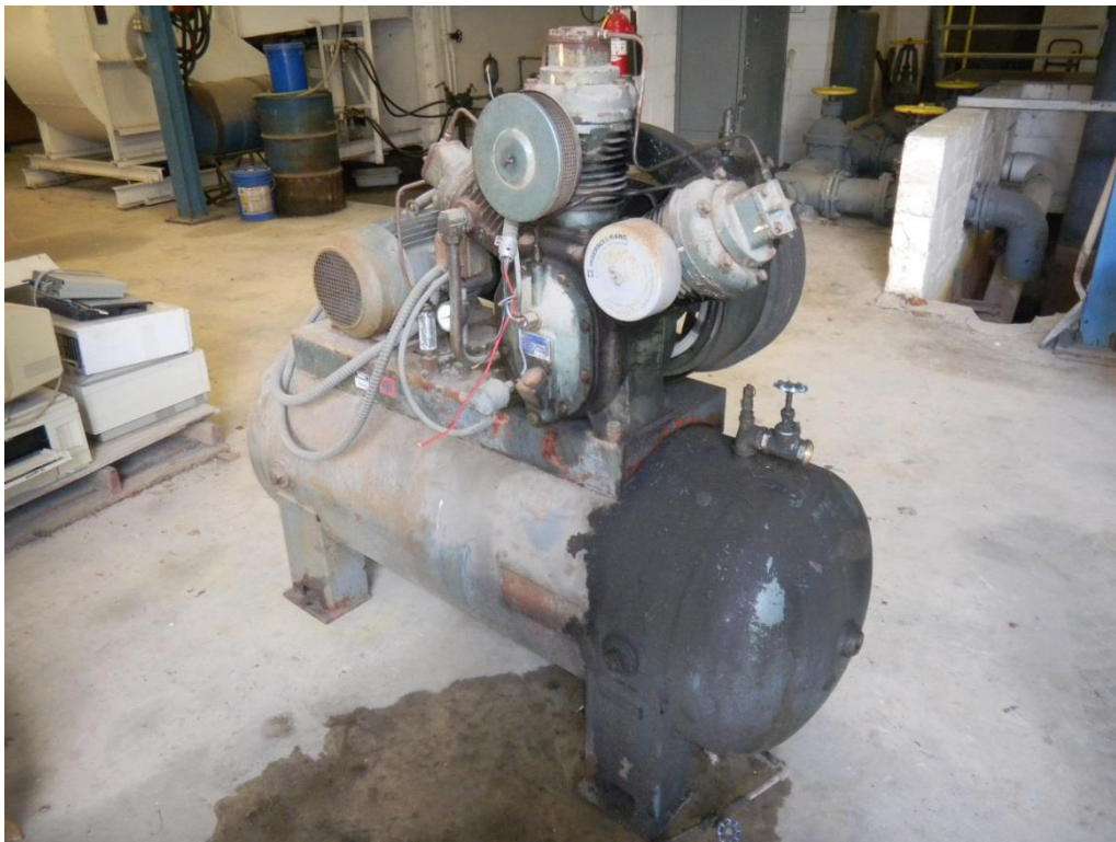
Figure 3-8. Old, existing air compressor.
