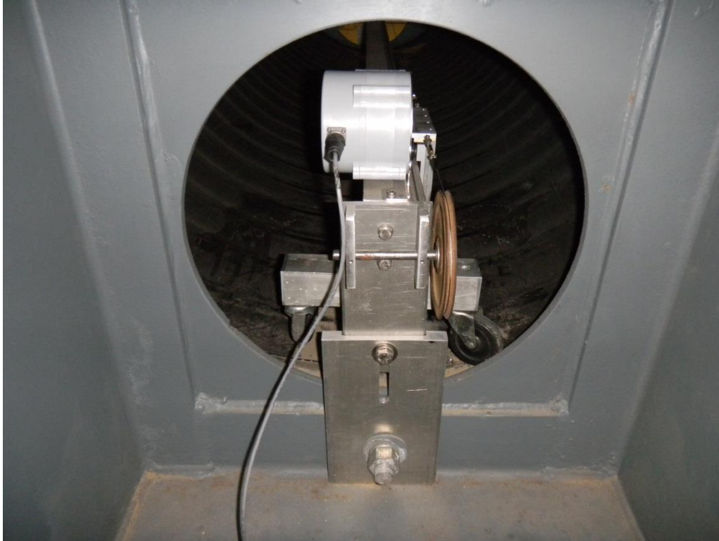
Figure 3-7. Installed laser profiling system.
