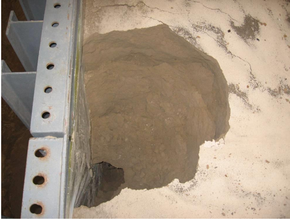
Figure 8-20. Top view of void formed above HDPE pipe end.
