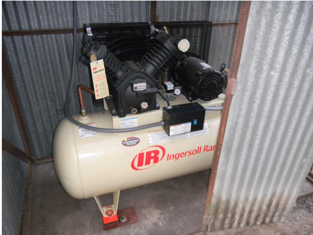
Figure 3-9. New, replacement air compressor.
