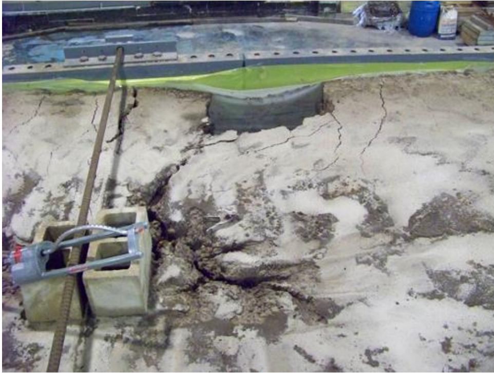
Figure 9-10. Void formed from flexible membrane breach
