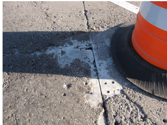
Figure 123 – Wearing surface damage at intersecting panels
