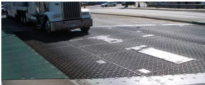
Figure 7 – Damaged and repaired existing steel grid deck
