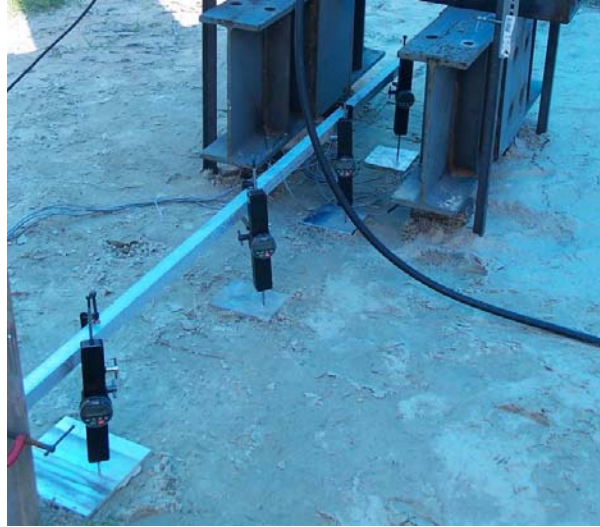
Figure 4-30 Digital dial gages for soil deformation monitoring.
