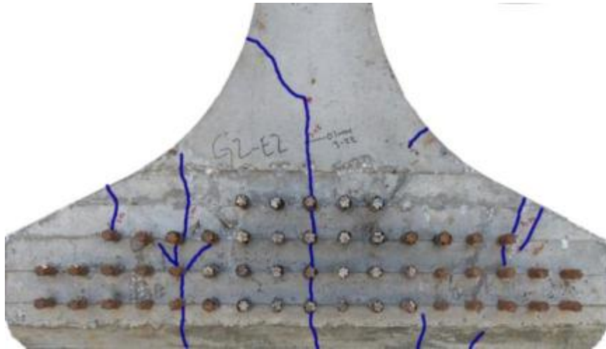
Figure 53–Flange splitting in experimental girder
