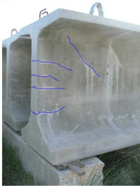
Figure 1–Web splitting cracks (enhanced in blue)
