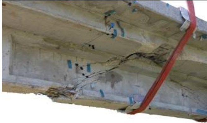
Figure 16–X7 punching failure bottom view
