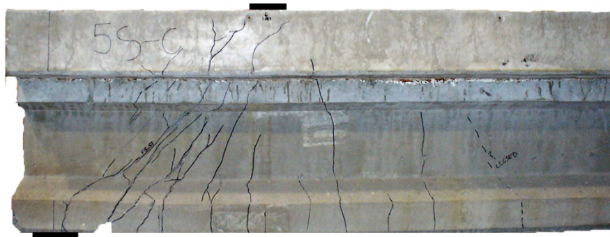
Figure 20–Flexural failure mode (B5S-C)
