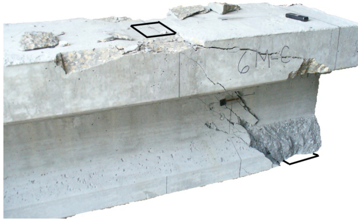
Figure 19–Bond-flexure failure mode (B6M-C)
