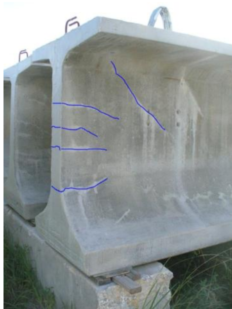
Figure 18–Web splitting cracks (enhanced in blue)
