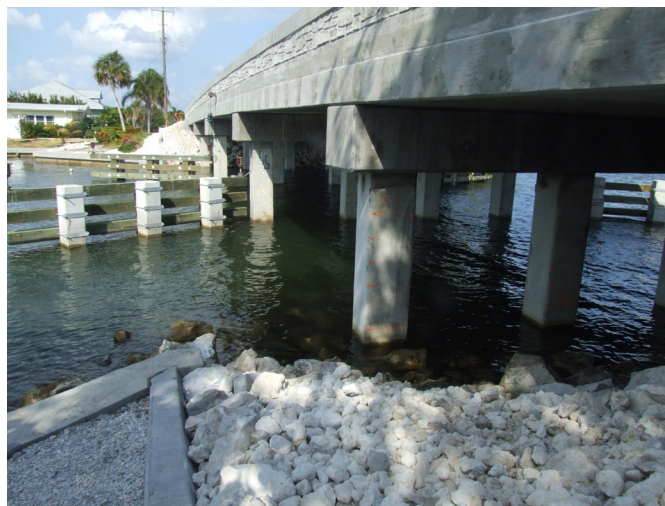
The piles that support the Key Royale bridge, studied in this project, are constantly subjected to the effects of salt water.
