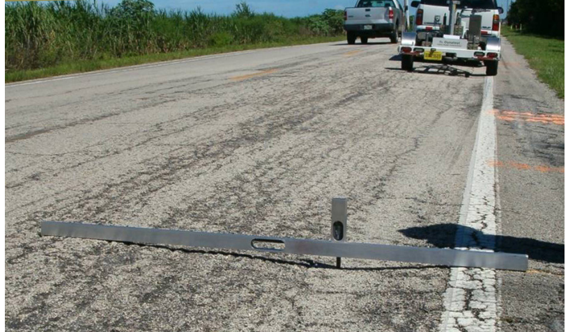
Foreground: A straight edge placed on the pavement measures the rut depth along State Road 15/U.S. 98 in Palm Beach County. Background: A falling weight deflectometer (FWD), mounted to a tow vehicle, evaluates the physical properties of pavement.
