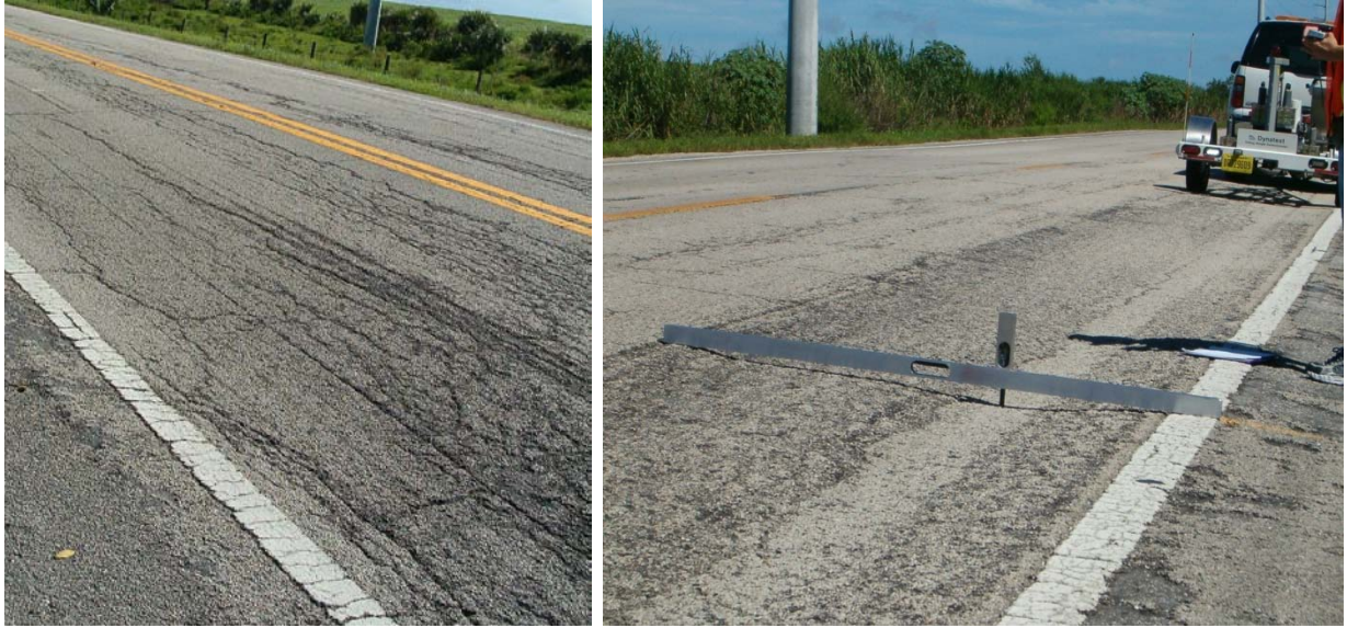
Figure 1.5: Alligator cracking and rutting along SR 15/US 98
