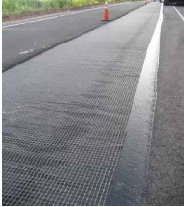
Figure 6.15: PetroGrid Mesh Separating due to Construction Traffic
