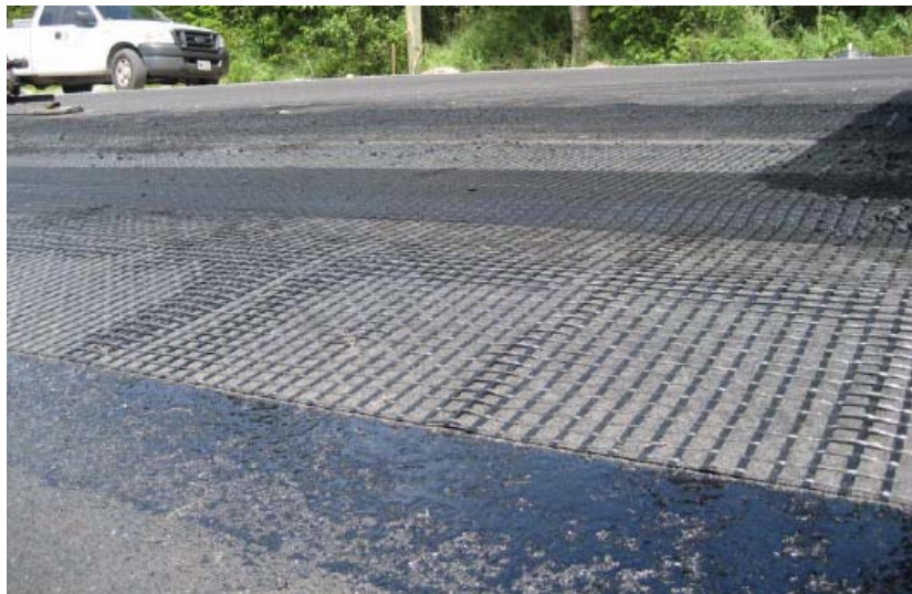
Figure 6.12: PetroGrid Mesh Separating from the Fabric
