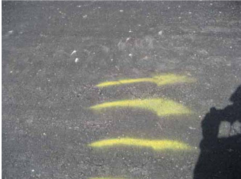
Figure 6.6: Hairline Cracks in PaveTrac Section 1.3S, ST 172+70
