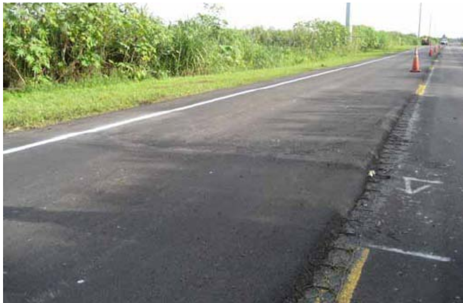
Figure 6.7: Rough Surface of 2.3S after 24 hours due to PaveTrac Curling
