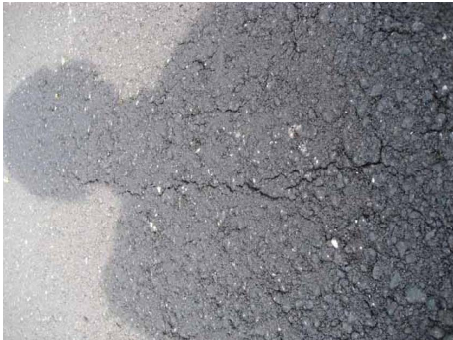
Figure 6.5: Transverse Cracks in PaveTrac Section 1.3S
