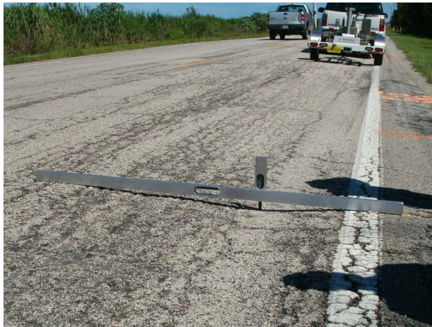
Figure 5.2: Rut Depth Measurement
