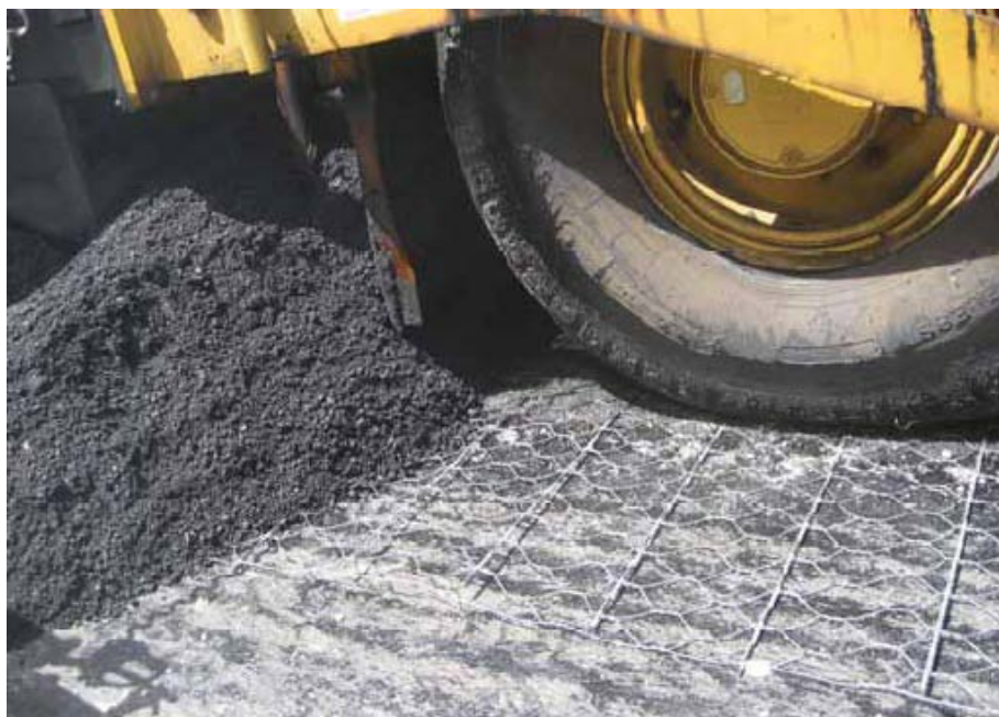
Figure 6.8: Additional Fasteners Resolve Wrinkles under Wheels
