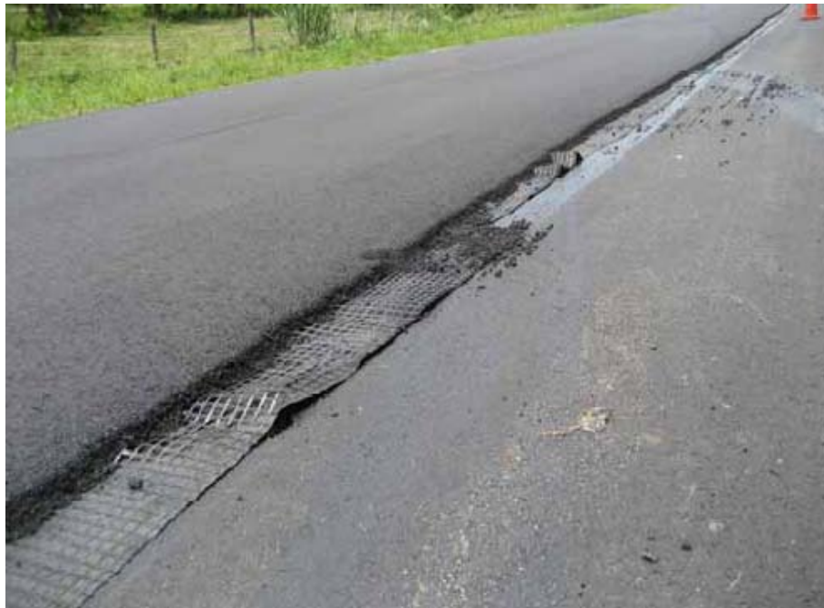
Figure 6.16: Wrinkles and Separations in the PetroGrid Material
