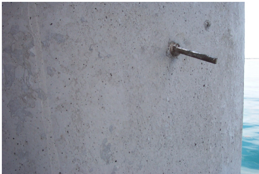
Figure 11: Photograph of the threaded stainless steel ground connection rod on the column of Pier 40W-East.
