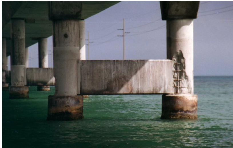
Figure 2: Seven Mile Bridge pier with thermal spray zinc applied to the two columns and strut.
