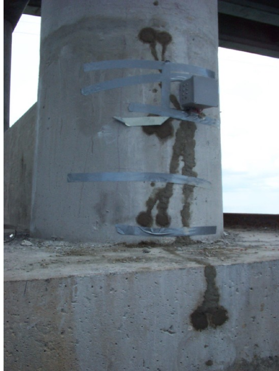
Figure 17: Photograph of Pier 40W-East upon completion of probe installation, wiring, and grouting.
