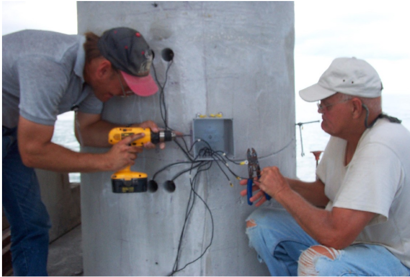
Figure 15: Photograph of the junction box installation and probe wiring on Pier 40W-East.
