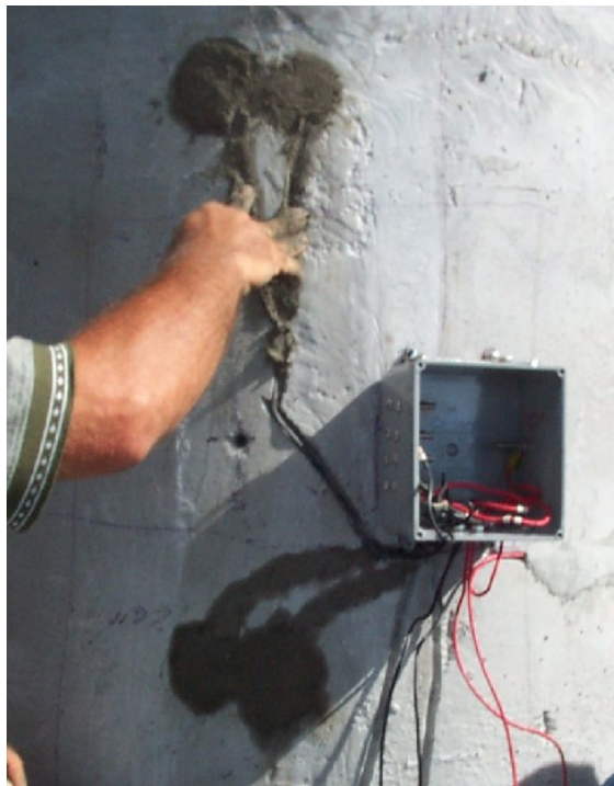
Figure 16: Photograph of the upper two core holes, grouted wire routing slots, and junction box on Pier 40W-East subsequent to installation.
