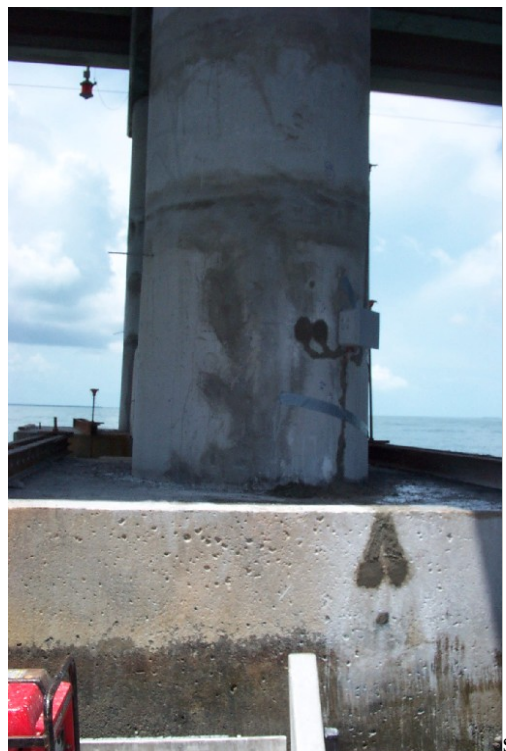
Figure 18: Photograph of Pier 39W-East upon completion of probe installation, wiring, and grouting.
