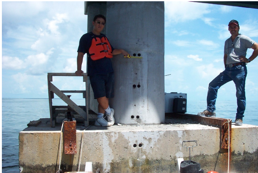
Figure 12: Photograph of Pier 40W-East of the Bahia Honda Bridge subsequent to drilling the four pairs of probe core holes.
