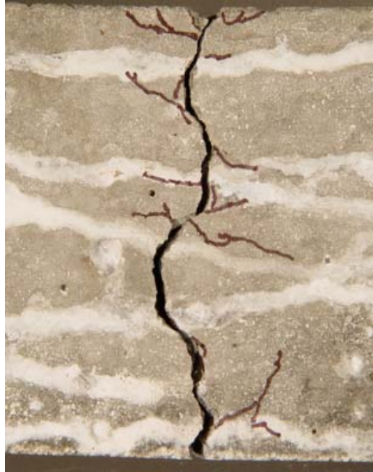
Figure VIII-48: Photograph of the bottom (tensile) face of the specimen of mix 54 showing the primary fracture (top to bottom) and highlighted ASR microcracks.
