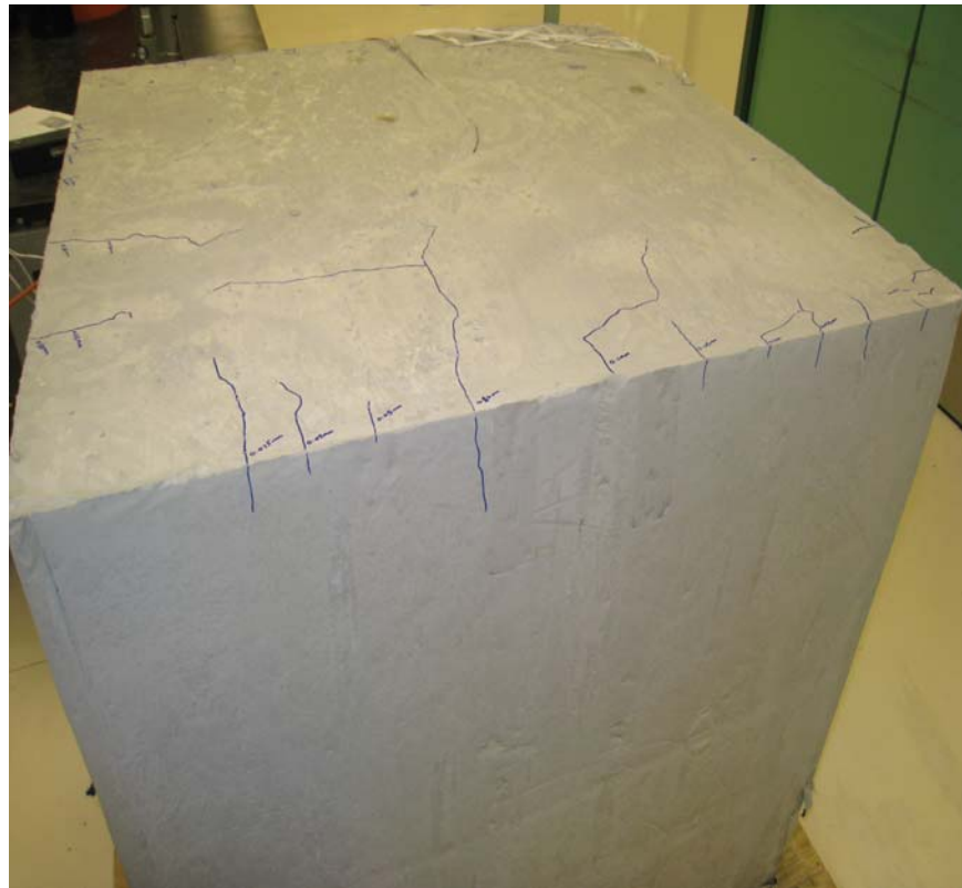
Figure 8-12. Top surface of experimental block containing Mixture 1 showing numerous cracks along the edges.
