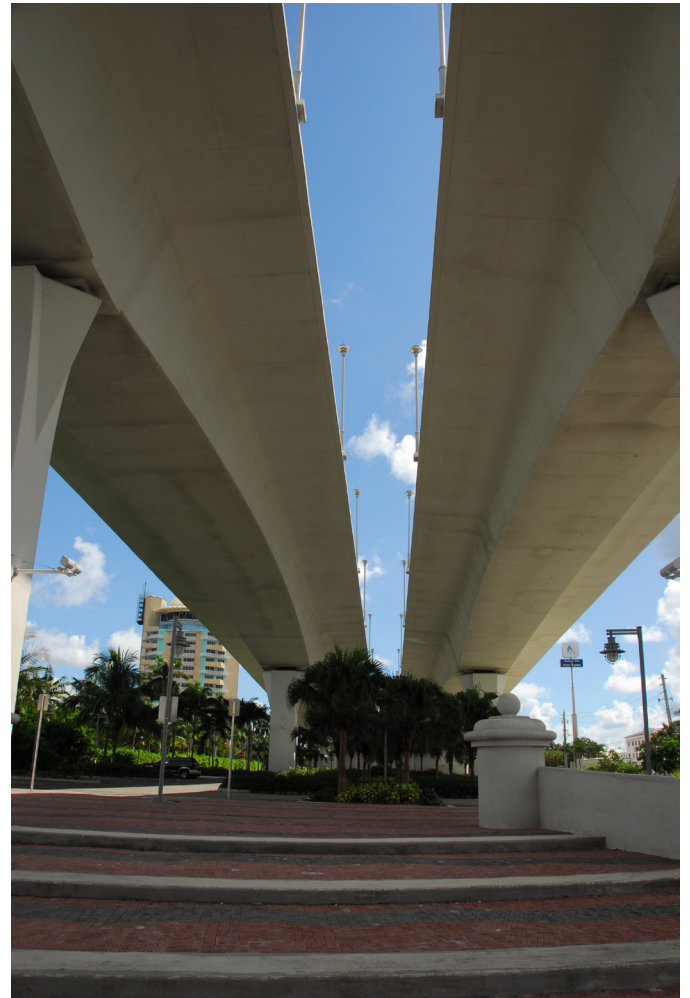
Large drilled shafts are necessary to support large bridges like this one in Ft. Lauderdale.
