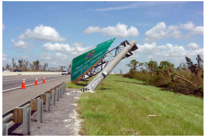
A failed cantilever sign structure
