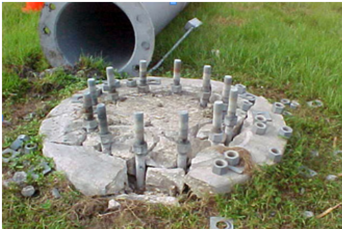
Damaged post base
