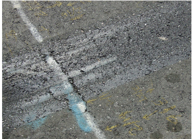
Tests on aged pavement produced lateral top-down cracks.
