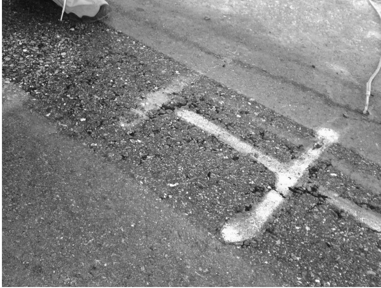
Figure 6.23 Cracking Induced at Paints in Section 1A
