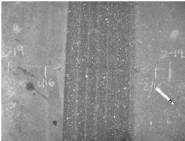
Figure 6.22 Transverse Cracking Developed in Section 1A
