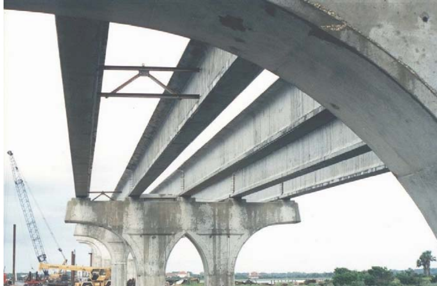
Figure 1.4 Florida bulb-tee girders placed on bearings (Vilano Beach Bridge, Florida / Photo credit: Florida DOT)
