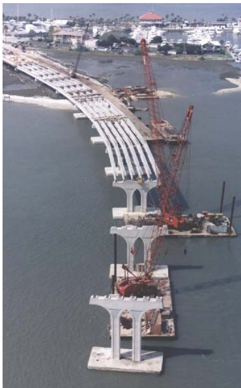
Figure 1.1 Construction of a girder-slab bridge using Florida bulb-tee girders (Vilano Beach Bridge, Florida / Photo credit: Florida DOT)
