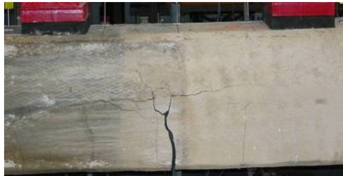
Figure 21 – Strand rupture of pile 44-3CP.
