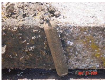
Figure 10 – Bulk zinc anode on pile 21-4
