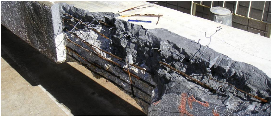
Figure 30 – Pile 44-3CP after excavation. Darker concrete is patch material placed during the 1994 repairs.
