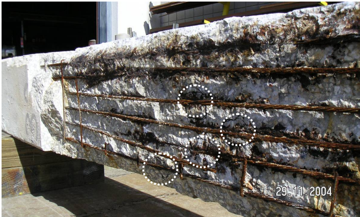
Figure 28 – Pile 32-3J after excavation. Wire breaks are circled.
