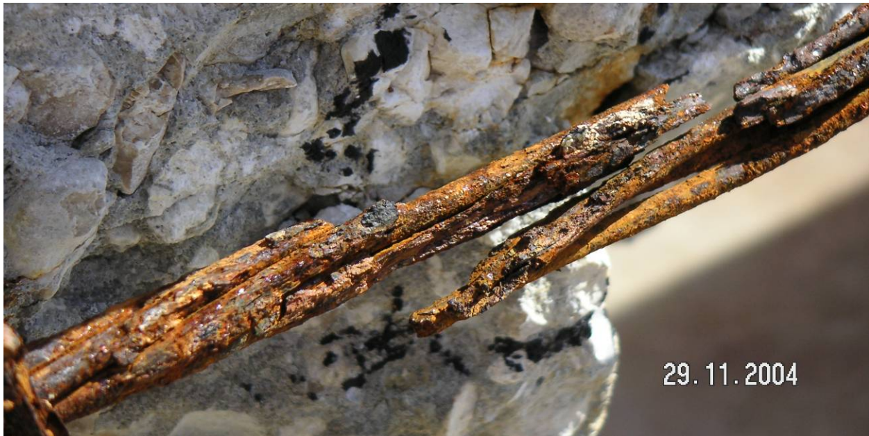
Figure 33 – Typical rupture pattern of severely corroded prestressing strand exhibiting fingernail splitting.
