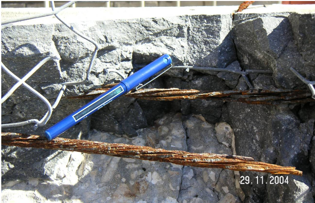
Figure 31 – Interface between existing pile concrete and patch material. Galvanized steel mesh was used in patch. Prestressing strand in foreground appears to have had significant section loss before repair.
