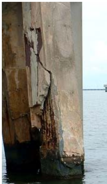
Figure 1 – Corrosion Damaged Pile
