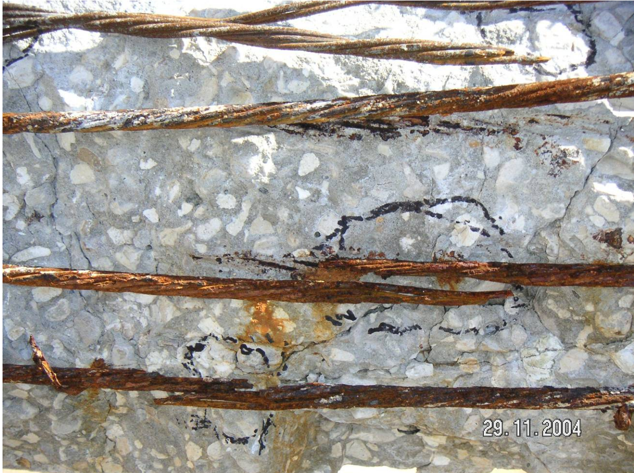
Figure 32 – Strand in bottom of pile 44-3CP. Corrosion severity increases in intensity from top to bottom. Wire breaks are distributed along a major flexural crack in the more heavily corroded strands.
