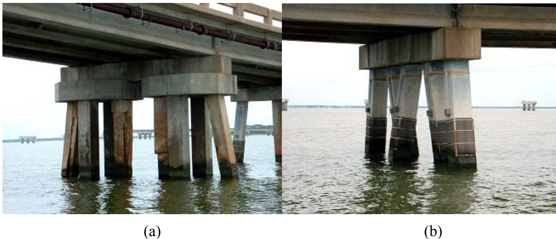
Figure 3 – Prestressed pile bents before bridge demolition. (a) “crutch bents” installed to relieve piles damaged by corrosion (b) cathodic protection system on existing piles
