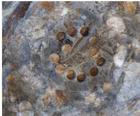
Figure 40 – Prestressing tendon from cylinder pile. Note grout surrounding wire with no evidence of conduit.
