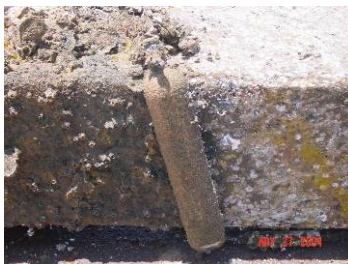
Figure 10 – Bulk zinc anode on pile 21-4
