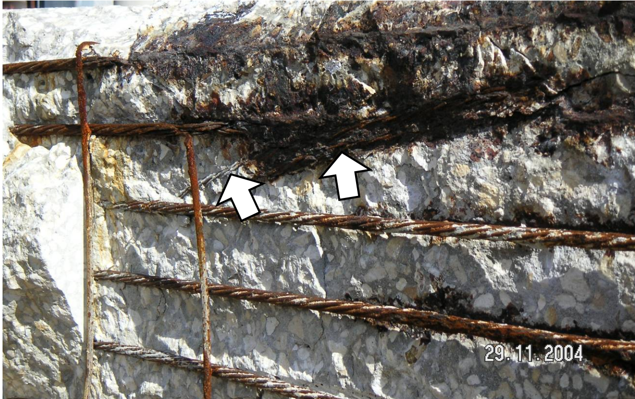
Figure 29 – Severely corroded strand from pick up point on Pile 32-3J. Prestressing strand in this area has been completely consumed by corrosion. Moderate to severe corrosion on the remaining strands as they enter the splash zone.
