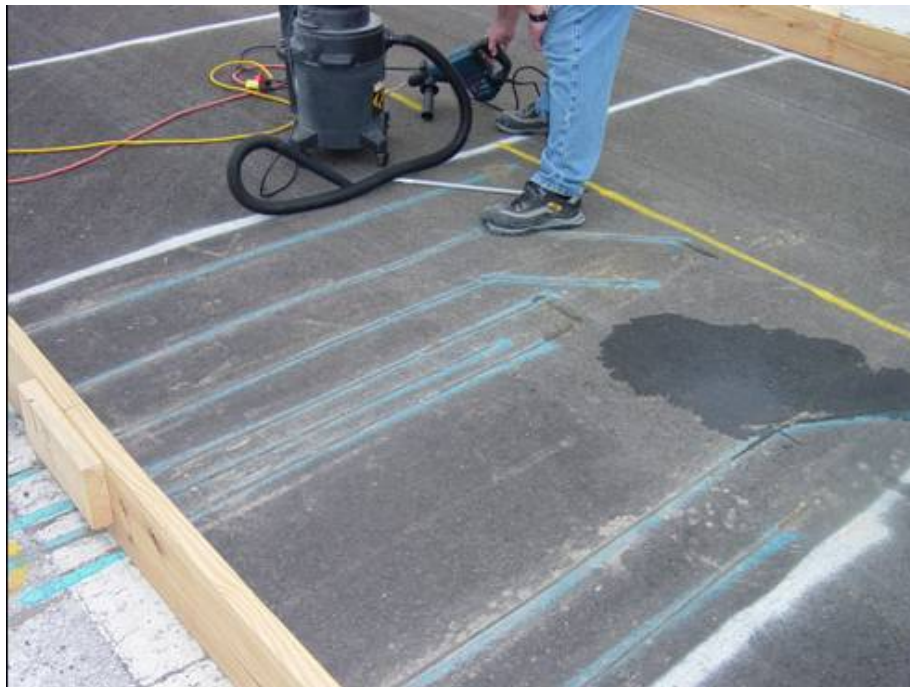
Figure 3.21. Grooves on Asphalt Surface for Placement of Strain Gages and Thermocouples Cables in Phase II.
