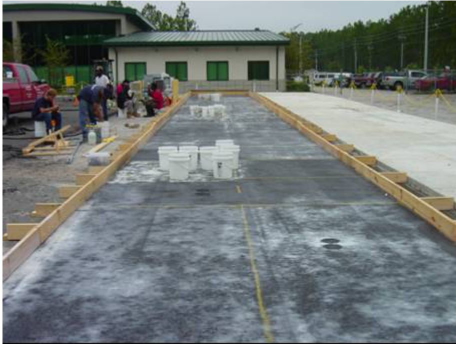
Figure 3.22. Asphalt Surface with White Curing Compound Before Concrete Placement in Phase II.
