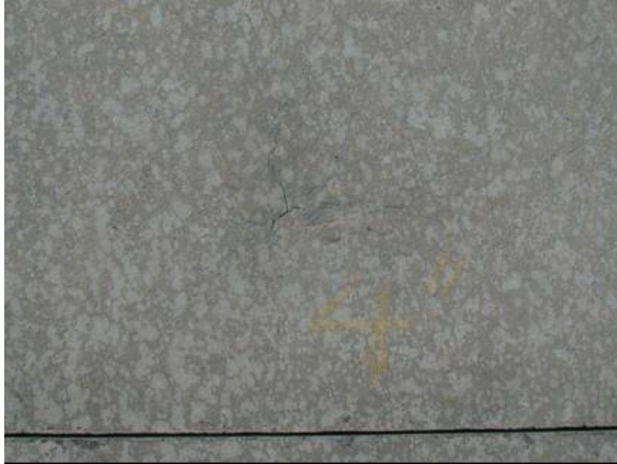
Figure 6.2. Shrinkage Cracks on a 4-inch Test Slab in Phase I-a.
