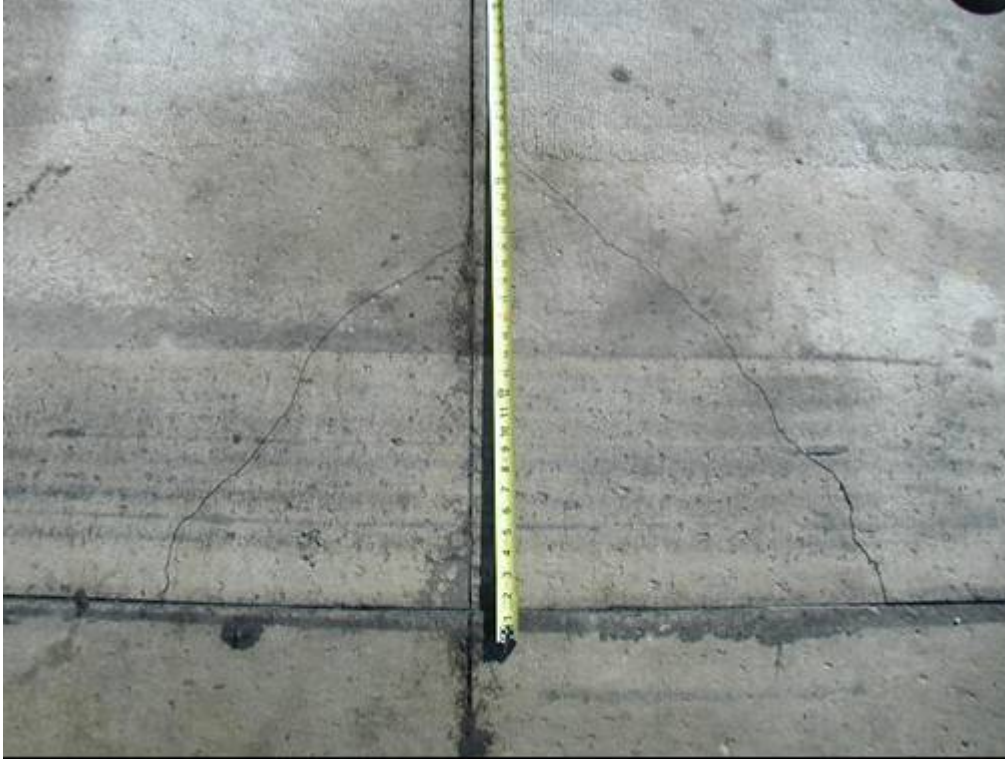
Figure 6.1. Corner Cracks on 4-inch Slabs in Phase I-a after 21-kip Wheel Loads.
