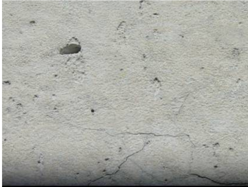
Figure 6.4. Shrinkage Cracks on a 6-inch Concrete Slab in Phase I-a.
