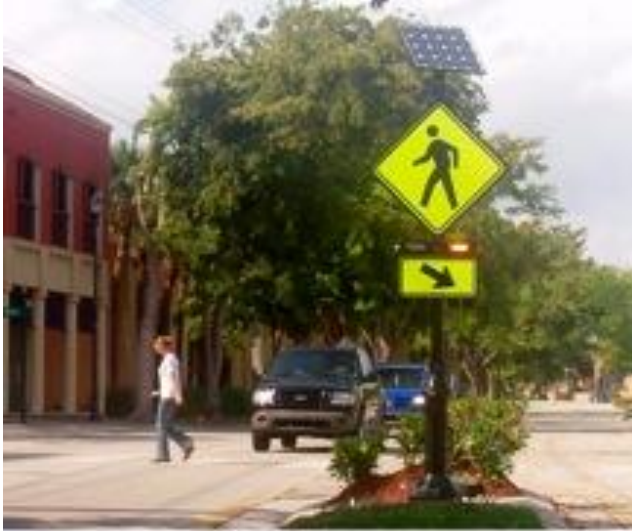
Figure 3.10 Picture of Rectangular LED Rapid Flashing Beacons
