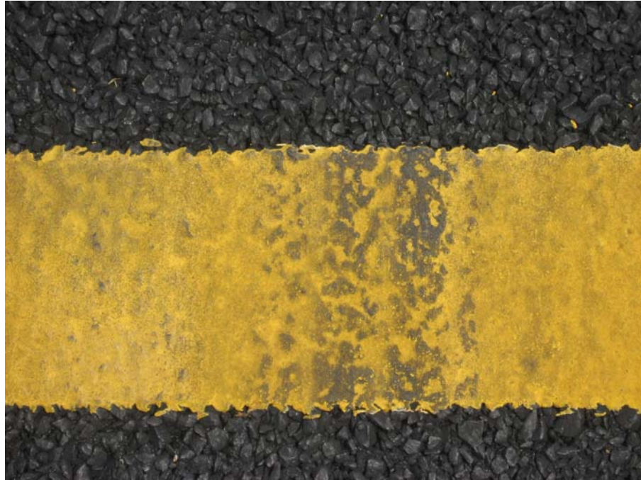
Figure 3-1. Wheel Tracking of Asphalt on to Surface of Pavement Marking (Product: R, Color: Yellow, Glass Beads: No)
