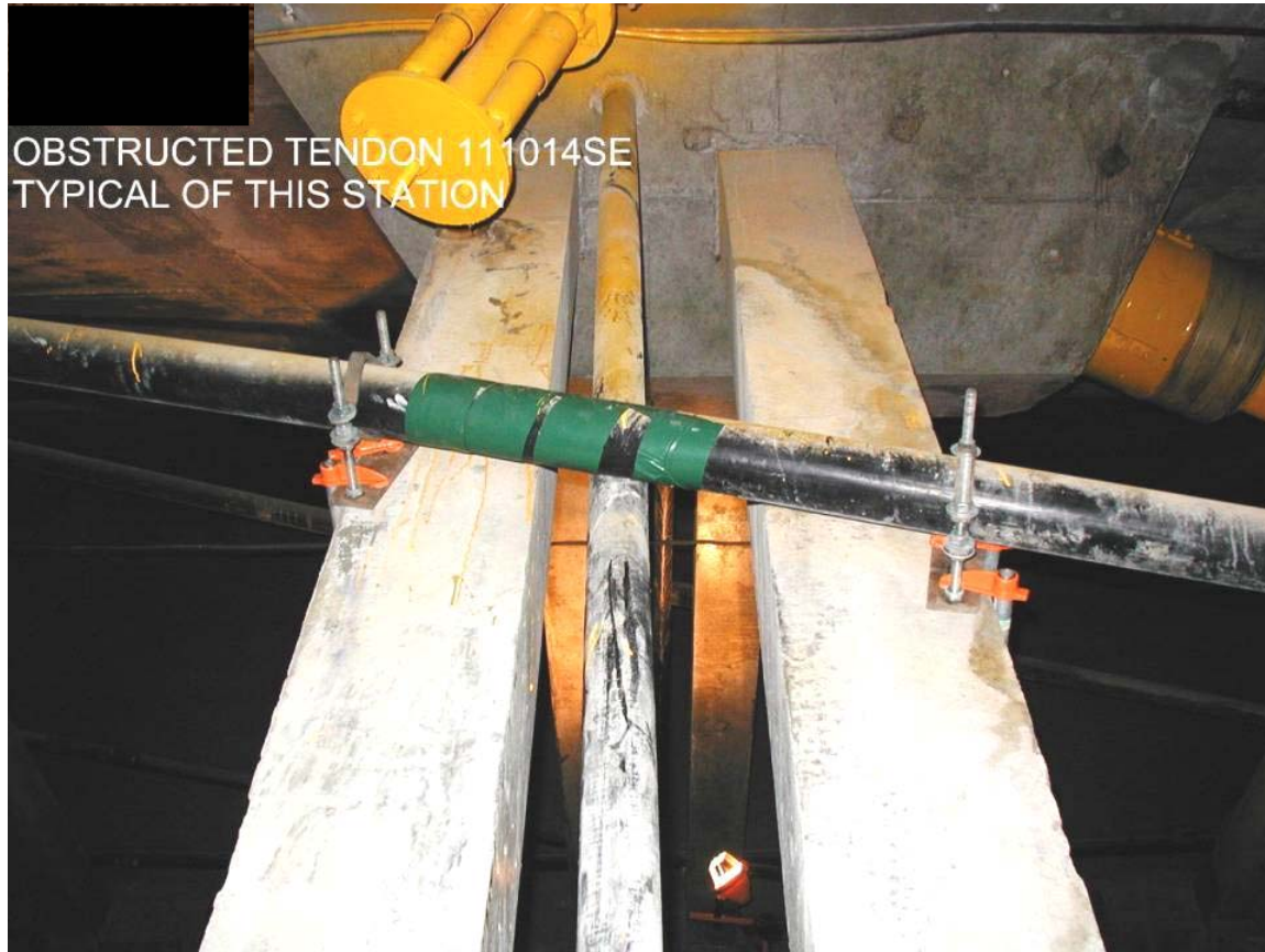
Figure 1. Example of Type 306 tendon (left to right) obstructed by touching a Type 014 tendon. Elevating frets are placed on each strut lifting the Type 306 tendon slightly so it clears the other tendon. The Type 014 tendon is then completely unobstructed and tested normally. Vibration testing of the Type 306 tendon is conducted on the side to the right of the right fret, with tension calculated using a specialized procedure. S is to the left.
