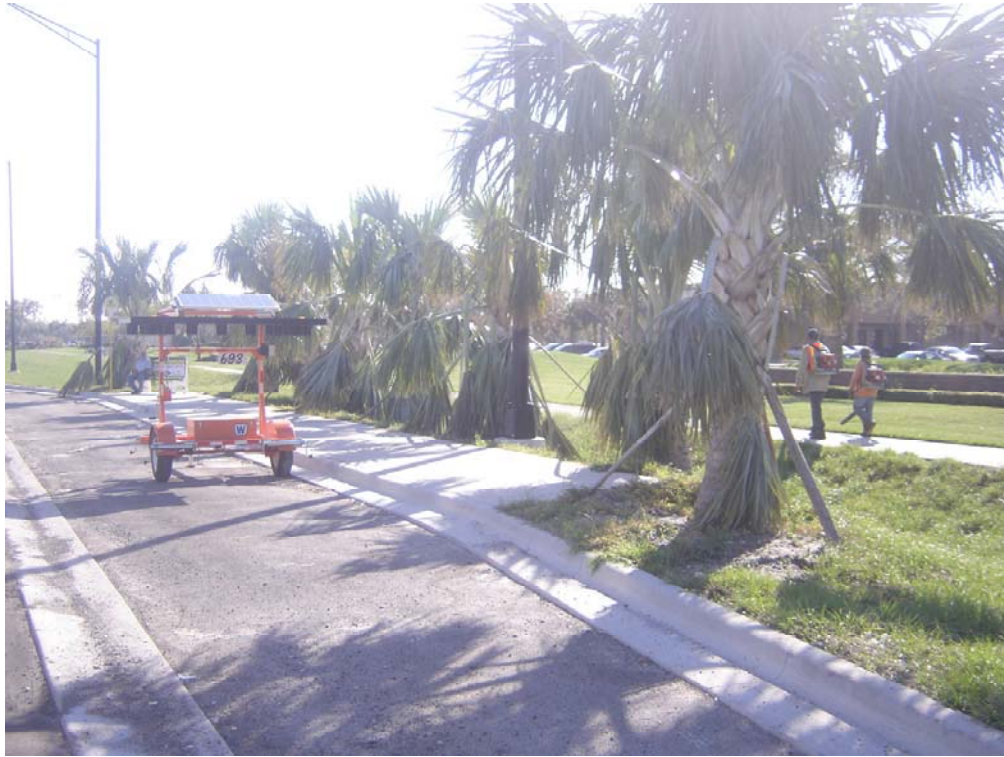
Figure 3.12. Pay Item No. 522-1 “Sidewalk Conc. 4 in” near the Pay Item 334-1-12 “SuperPave rebuild” GPS-measured on Nov. 10, 2005: Southbound View
