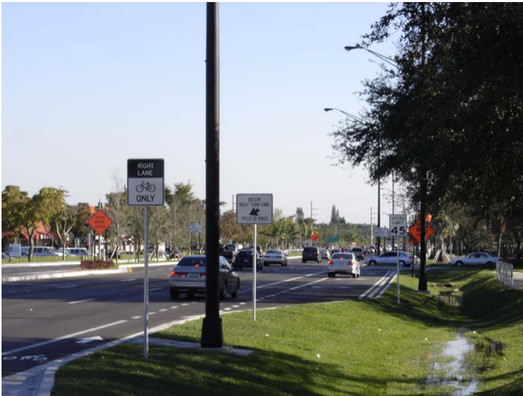
Figure 3.4 Pay item 520-1-10 “Curb & Gutter Conc. Type F with Signs and Light Poles GPS-Measured on Feb. 11, 2005: Southbound View
