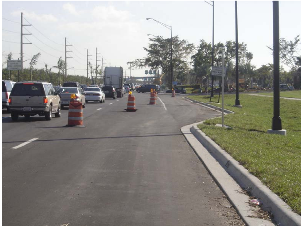
Figure 3.14 Pay item No. 520-1-10 “Curb & Gutter Conc. Type F” GPS-measured on Nov. 10, 2005: Southbound View
