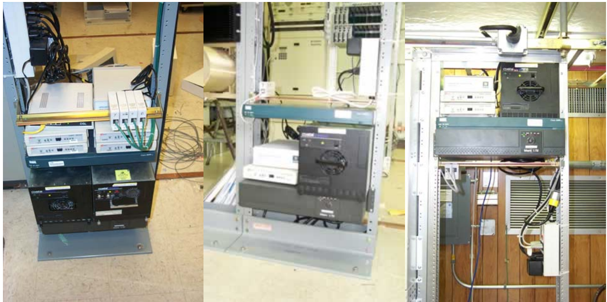
Figure 2: Typical installations of the original data network and acquisition equipment for the RWIS Research Facility.
