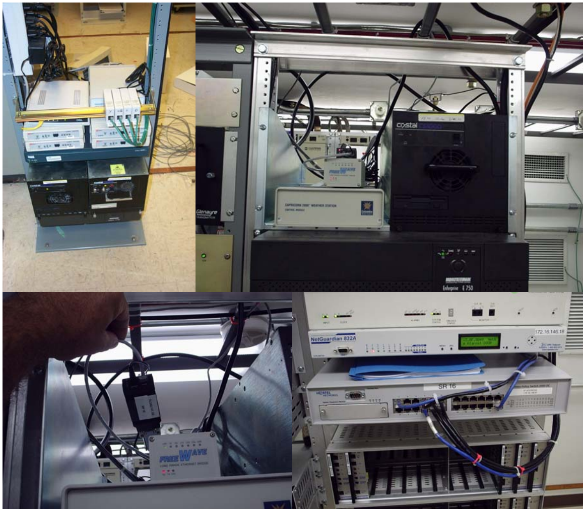
Figure 22: The original data acquisition and networking configuration (incorporating the required CSU/DSU units and a Cisco Router) is shown in the upper left picture. The upgraded configuration is shown in the upper right photo. This new configuration no longer requires the CSU/DSU units or the router. UNF also upgraded the system to incorporate a Digi TS-1 (One Port) Serial Terminal Server (shown in the lower left photo) connected to the FDOT MAS Ethernet network switch (shown in the lower right photo) to improve reliability of the system..
