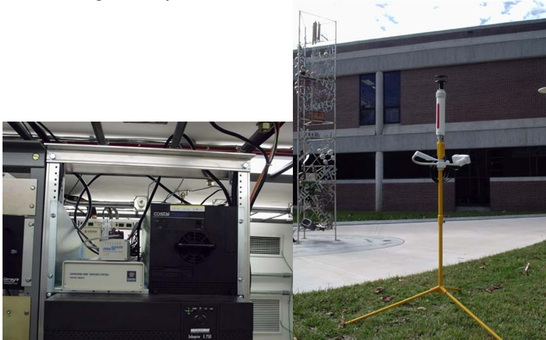
Figure 10: 900 MHz radio installed in SR16 MAS Tower (left) to provide communications with the evacuation bridge wind sensors and portable between-tower stations such as the portable station (shown on the right) that is being used in the iFlorida RWIS demonstration project.
