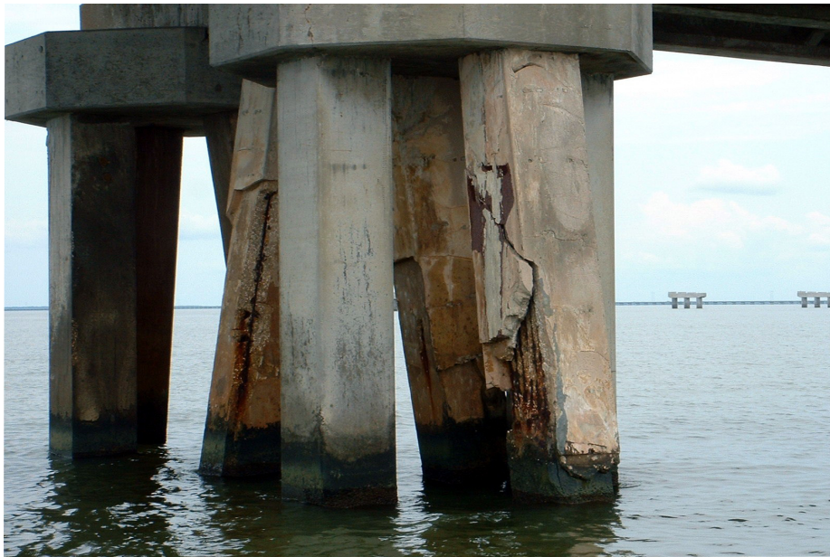
The results of corrosion are visible in the spalled concrete and exposed corroding steel reinforcement.
