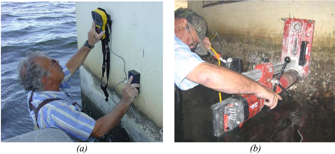
Figure 90. Bridge Coring Process. a) Locating Reinforcing Steel, b) Locating Drill for Coring.
