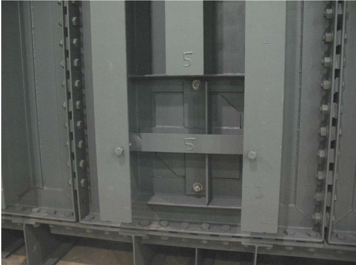
e) Pipe Access hole and cover
