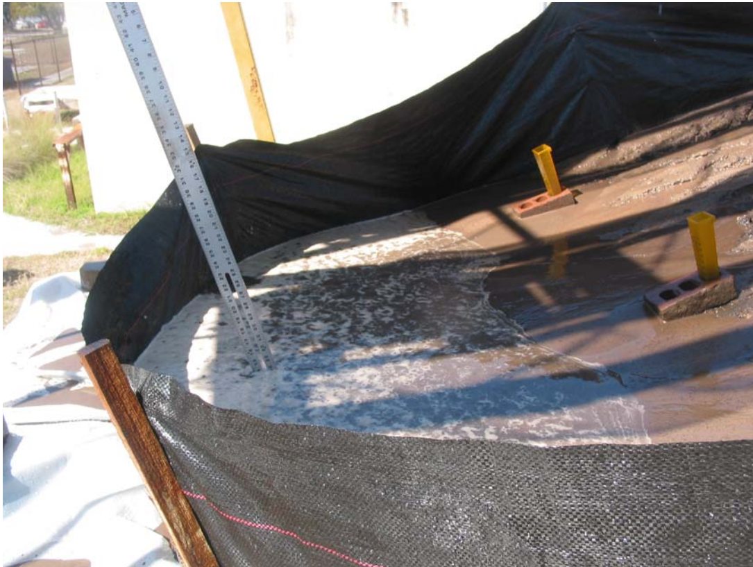
Figure 17 After a 3 Inches per Hour Rain Event, the Silt Fence Remains Stable.
