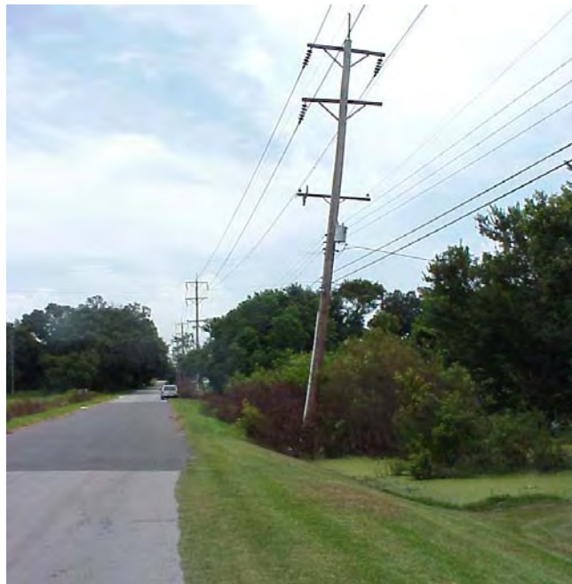
Leaning Power Pole at Glen Harwell Test Site
