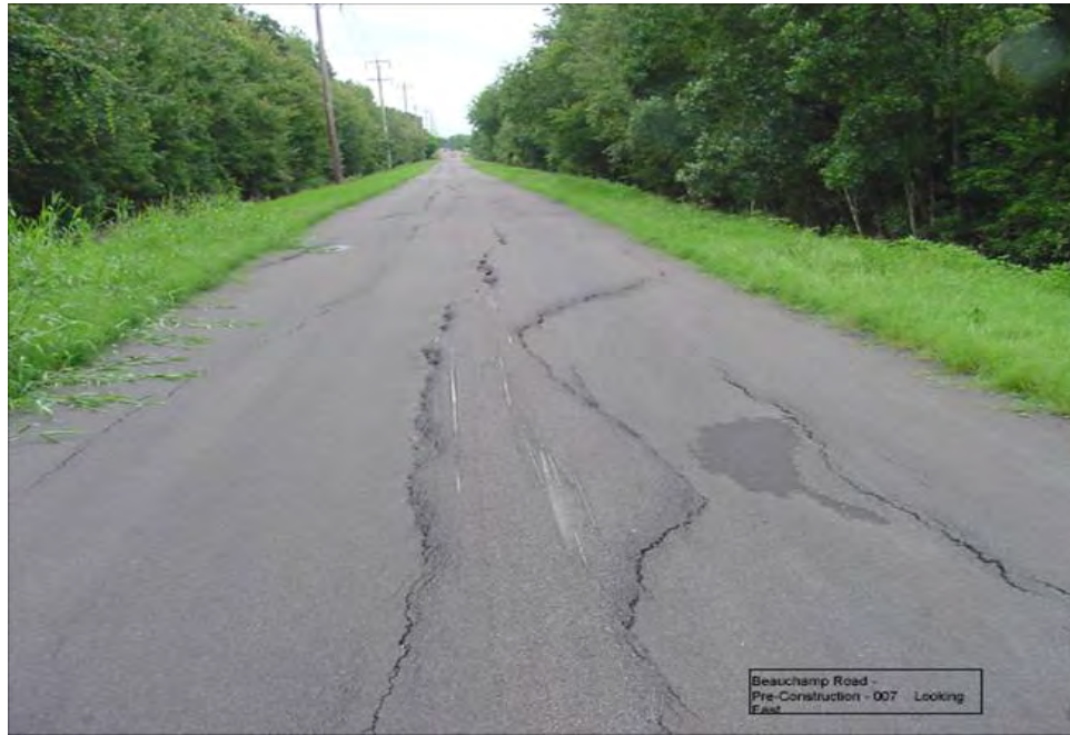
Beauchamp Road Test Site Prior to Repair
