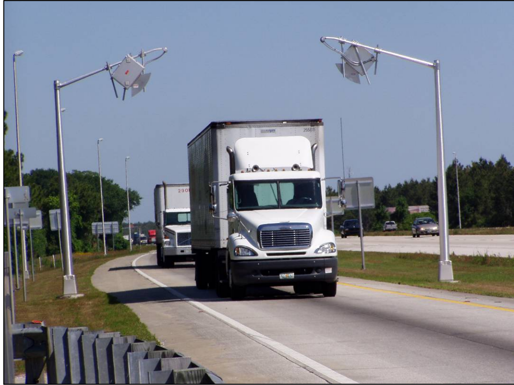
Figure 10: Laser system deployment at the entrance of WIM
