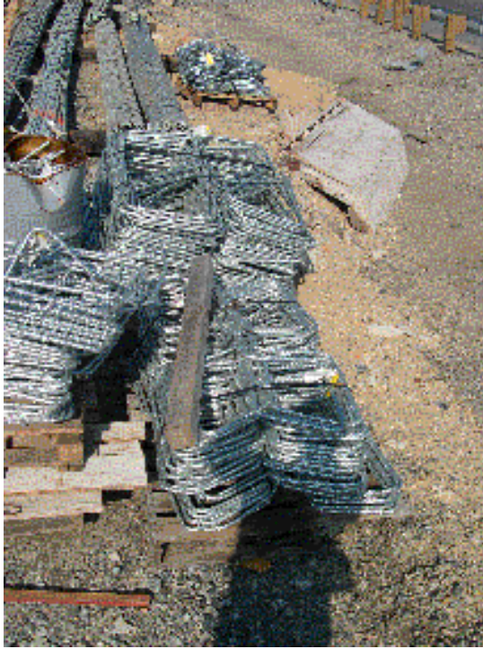
Figure E-5: Fabricated galvanized bars at the Frontage Road Bridge job site.
