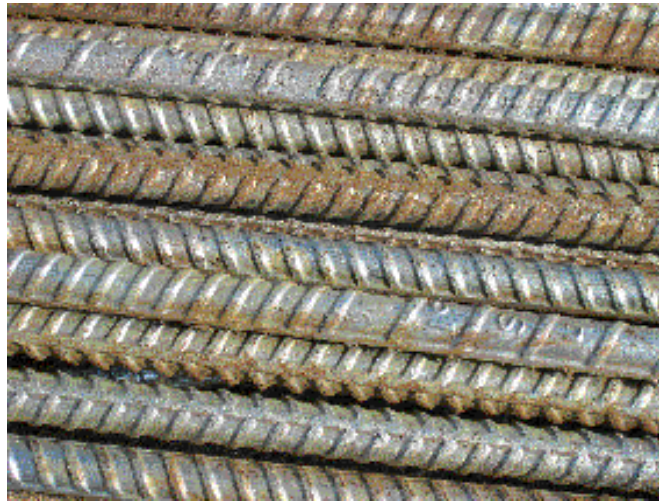
Figure E-9: Photograph of deposits on the galvanized reinforcing bars.
