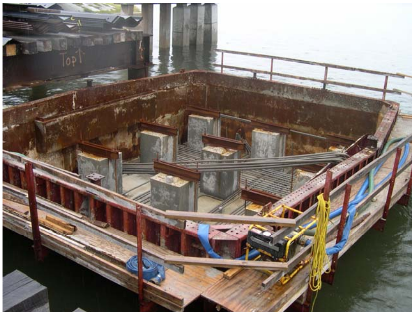
Figure B-2.4: Photograph of formwork, piles, and reinforcement being placed in the footer of pier number 12.
