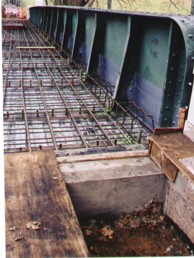
Figure A-3: General view of in-place reinforcement, girders with studs, curb, and bulkhead.
