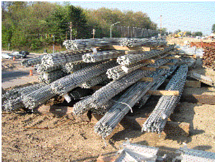
Figure E-6: Photograph of stored galvanized bars at the Brown Avenue Bridge job site.
