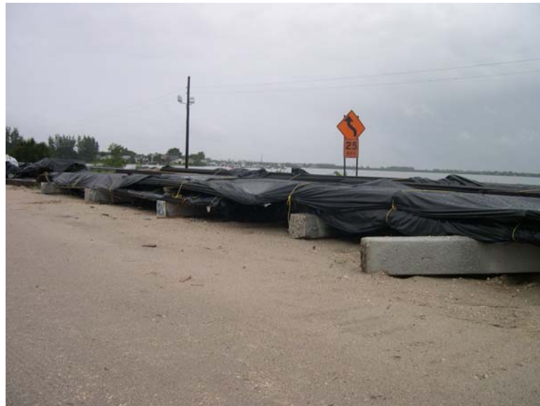
Figure B-1.5: Photograph of stored MMFX-II™ reinforcing steel at the job site.
