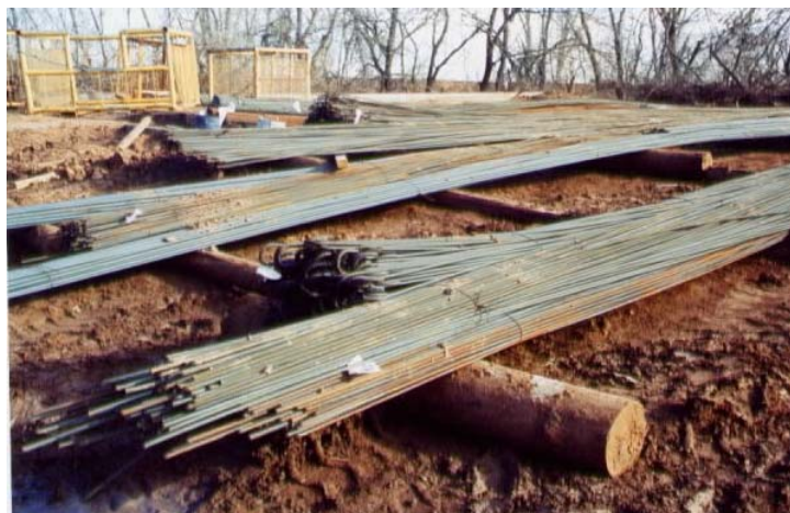
Figure F-6: Photograph of stored bars on timbers at job site.
