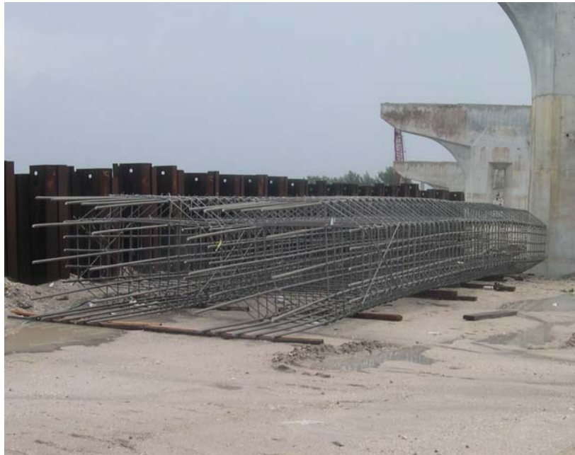
Figure B-2.6: Photograph of 2201 ss reinforcement cage for the column of pier number 11.
