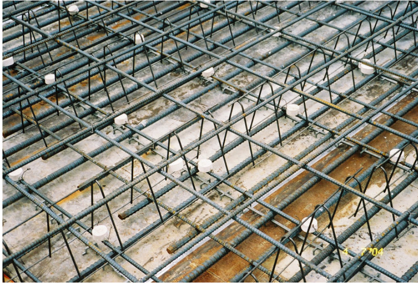
Figure G-6: Close-up view of discrete galvanic anodes on in-place Span 1 black bars.
