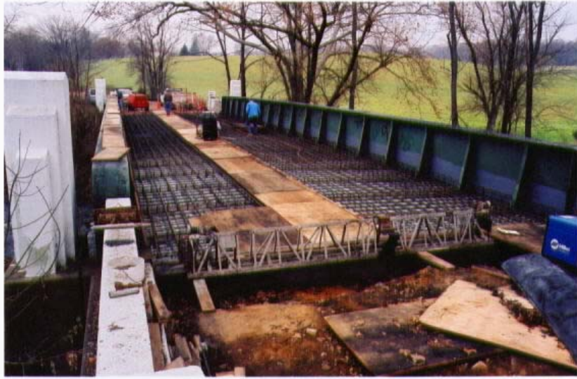
Figure A-2: Photograph of the bridge deck with MMFX-II™ reinforcement in place.
