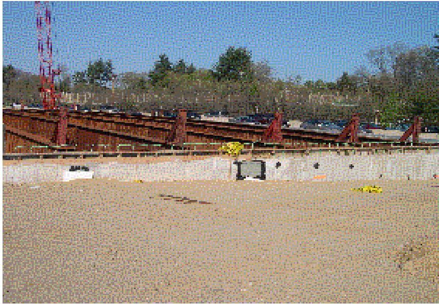
Figure E-2: View of the in-place girders on the Brown Avenue Bridge. Note ECR extending from the top of the backwall.
