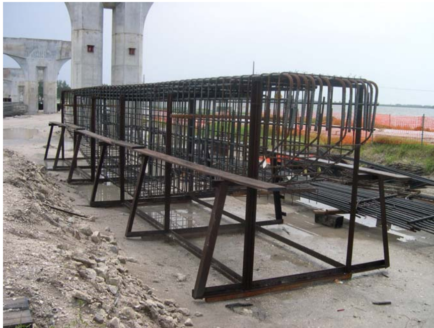
Figure B-2.8: Photograph of the conventional bar reinforcement cage for a hammerhead column cap.
