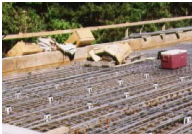
Figure D-5: Photograph showing cardboard packaged bent reinforcement details.
