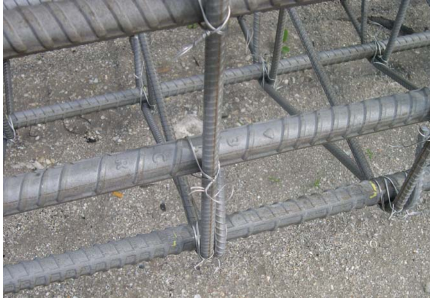
Figure B-2.7: Close-up view of a portion of the 2201 ss reinforcing bars in the column cage prior to placement in pier number 11.
