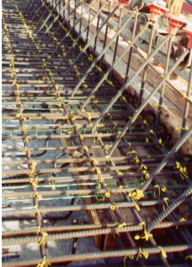
Figure F-4: Photograph of reinforcing steel as placed in the deck and parapet wall.
