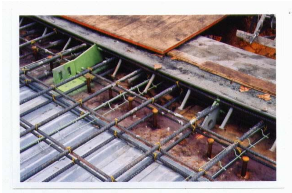
Figure A-4: Close-up view of reinforcing steel, girder with shear studs, gusset plate, and forming for bulkhead.
