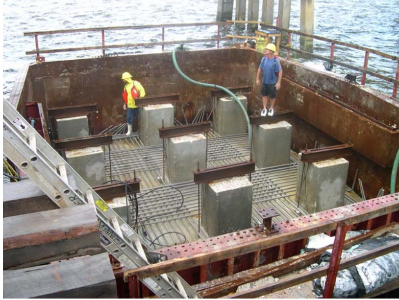
Figure B-2.3: Photograph of formwork, piles, and reinforcement being placed in the footer of pier number 12.
