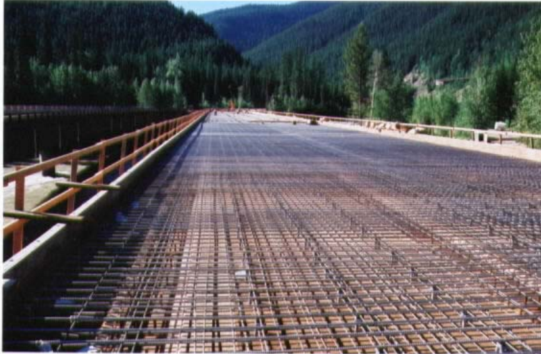
Figure D-1: View of deck with stainless steel reinforcement placement in progress.
