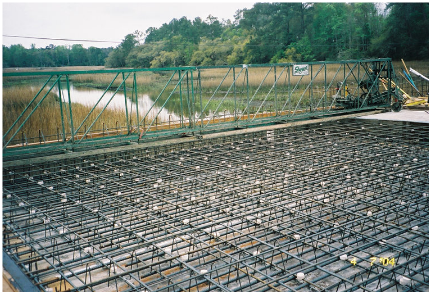
Figure G-5: View of in-place black bars (Span 1) along with discrete galvanic anodes.
