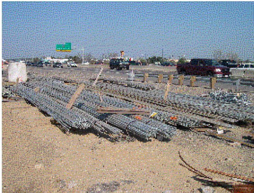
Figure E-4: Photograph of bundled/wrapped bars at the Frontage Road job site.
