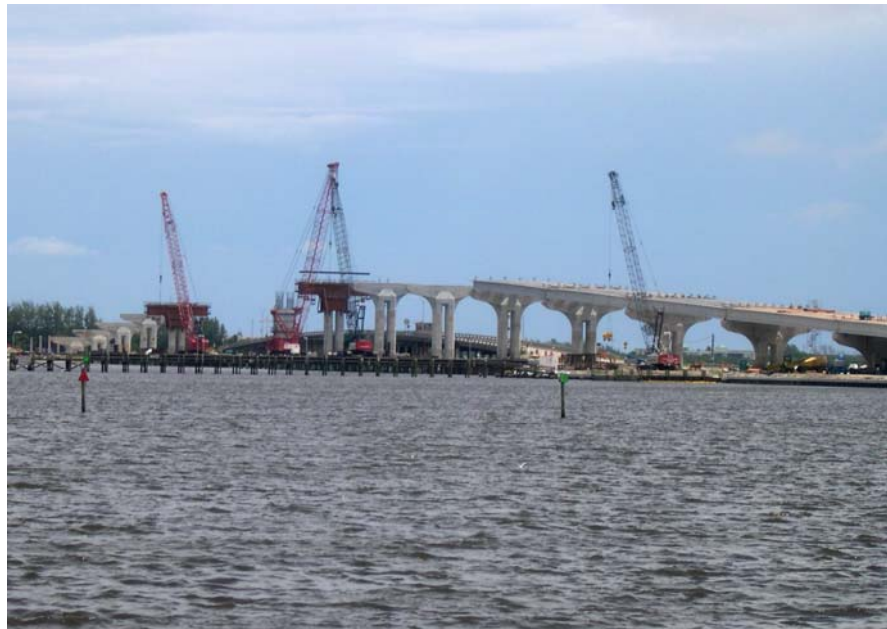
Figure B-2.1: Perspective photograph of the Jensen Beach Causeway Bridge under construction.
