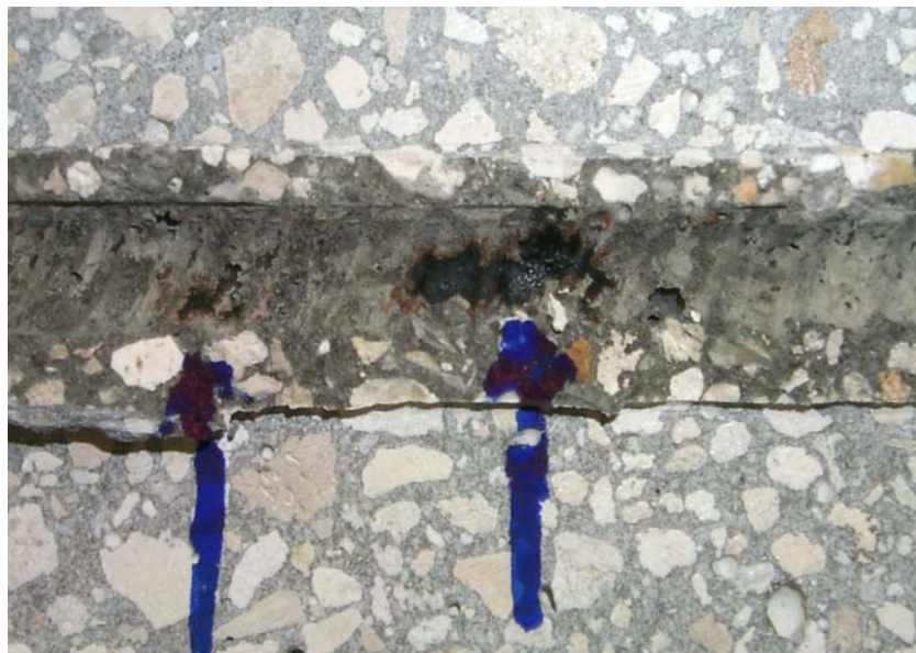
Figure 42: Photograph of corrosion on the rebar trace of Specimen 7.
