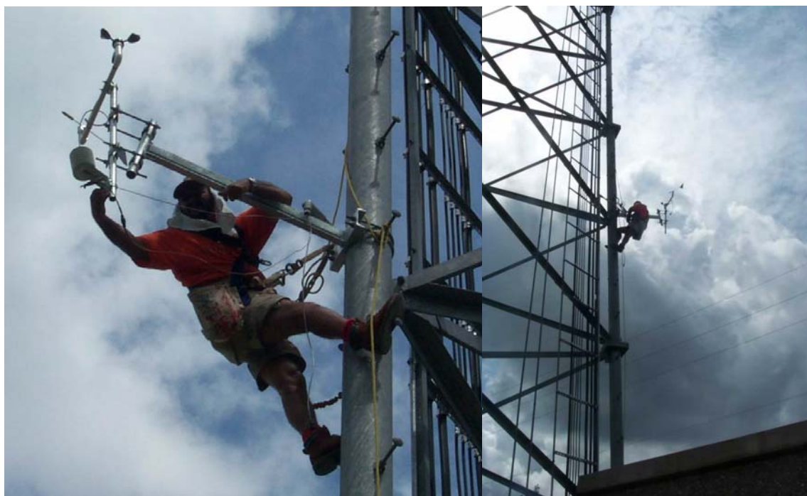
Figure 6: Typical installation of the “basic weather station” sensors for the prototype facility.
