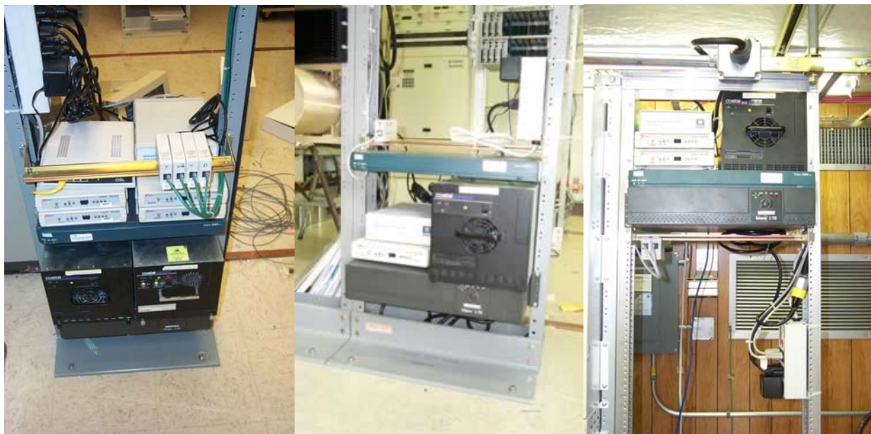
Figure 5: Typical installations of data network and acquisition equipment for the RWIS prototype facility.
